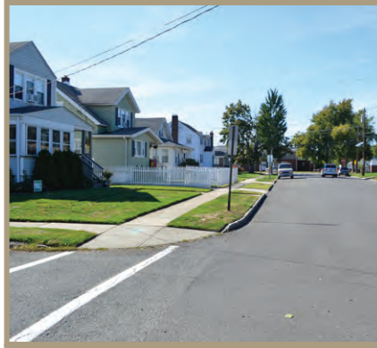
Figure 18. Non-compliant curb ramp.
