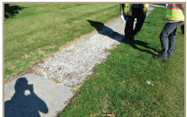
Figure 11. Missing concrete sidewalk section.
