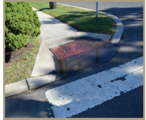
Figure 19. Puddling at base of ramp.
