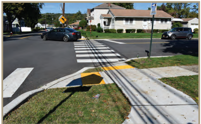
Figure 38. Crosswalks and ramps should be updated to match the intersection of Maple and Thompson.
