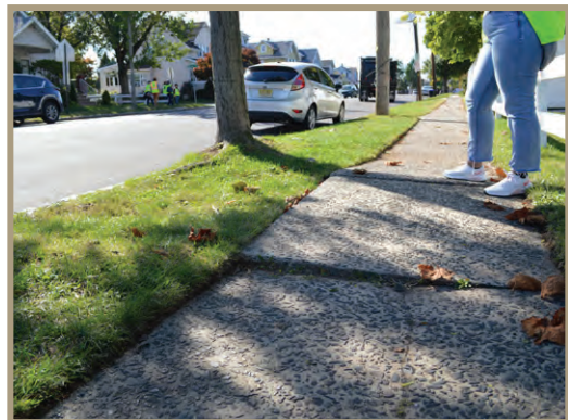
Figure 12. Sidewalk raised by tree roots.
