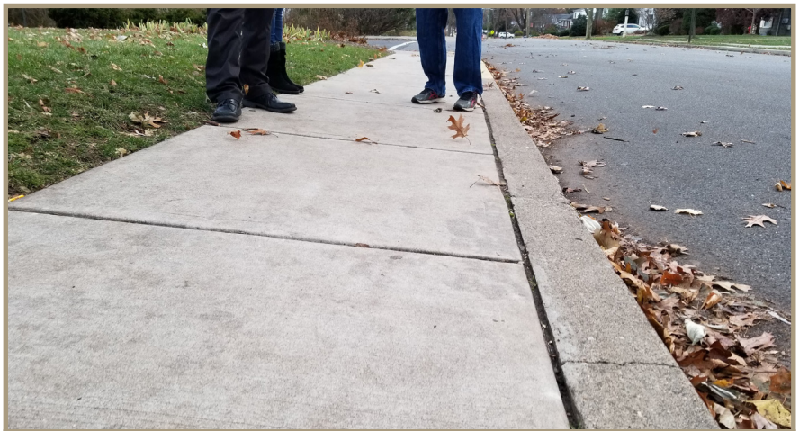
Figure 17. Sidewalk sloped towards roadway.
