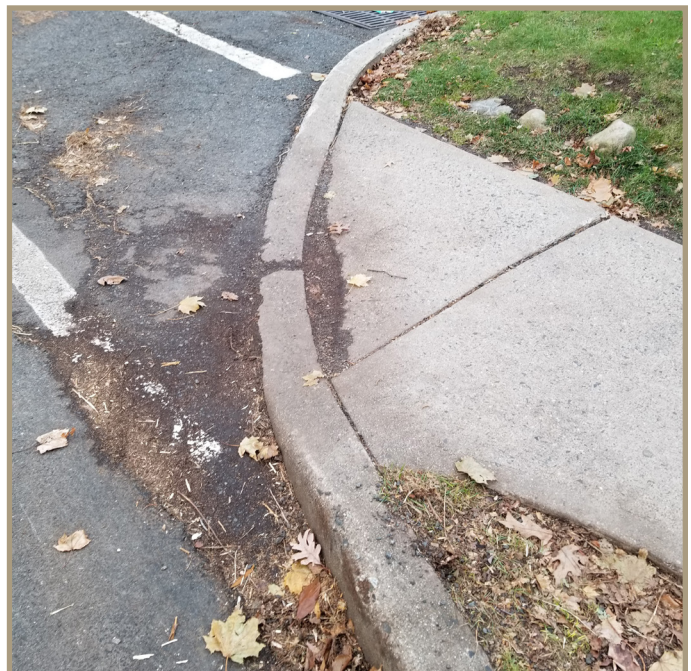
Figure 21. Ramps not ADA compliant along corridor.
