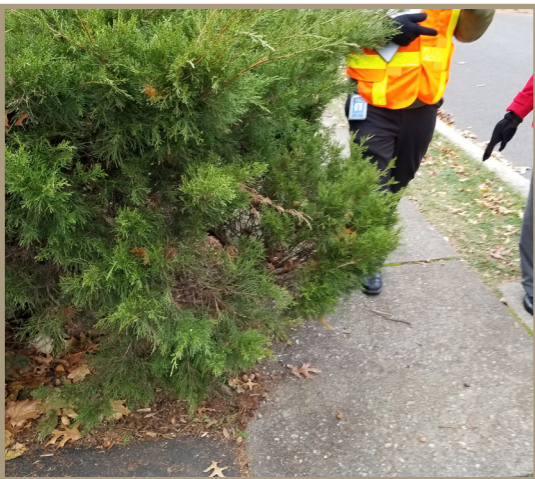
Figure 16. Sidewalk blocked by vegetation.
