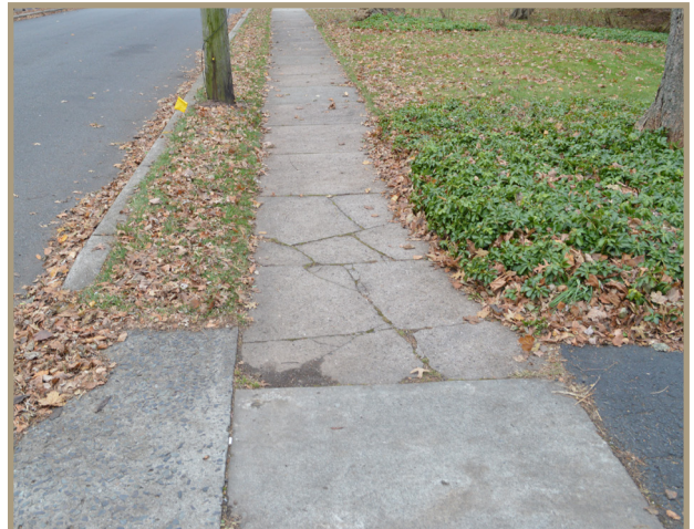
Figure 15. The corridor has continuous sidewalks on both sides, although cracking is apparent in parts.
