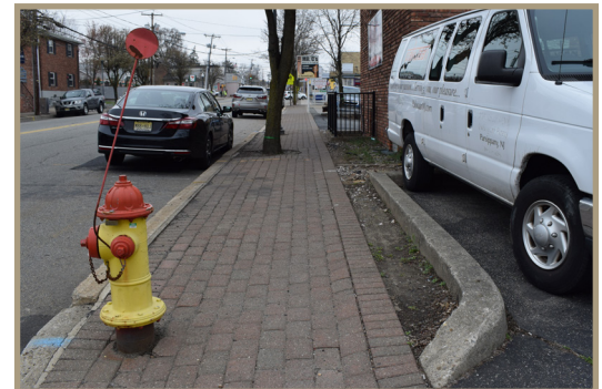
Figure 47. Sloping sidewalk and uncovered tree wells looking south on North Beverwyck Road, north of Lake Shore Drive.
