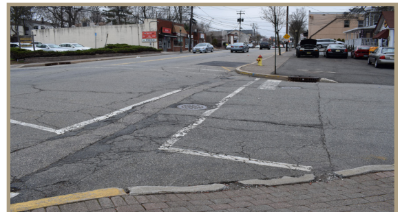
Figure 26. Missing curb ramp and steep, eroded ramp at the intersection of North Beverwyck Road and Minnehaha Boulevard, looking northward.
