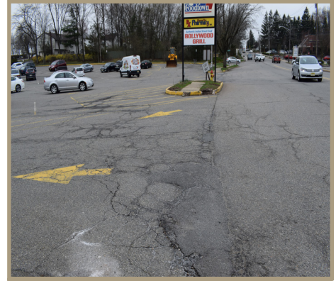
Figure 14. Missing sidewalks in front of Foodtown, looking south on North Beverwyck Road.
