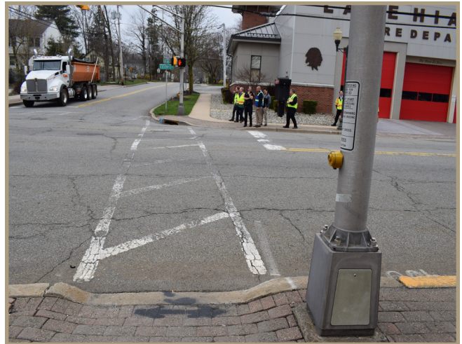
Figure 29. Fading crosswalk looking westward across North Beverwyck Road the intersection of Lake Shore Drive.
