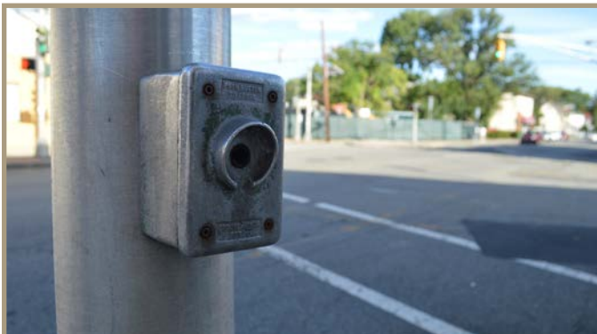
Figure 25. A non-functioning push button on a traffic signal.
