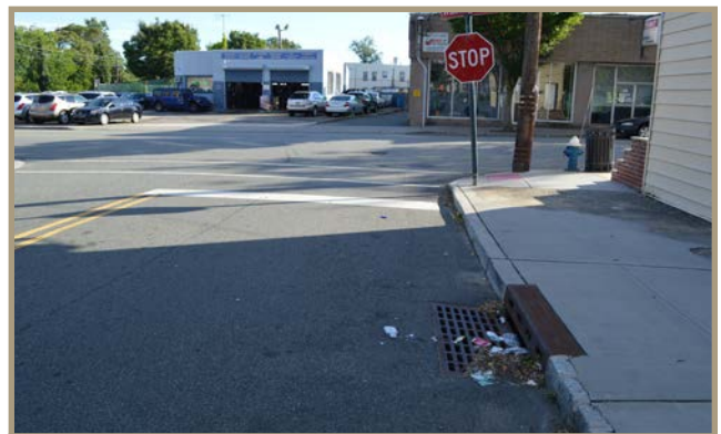
Figure 29. Trash collecting on a drain.
