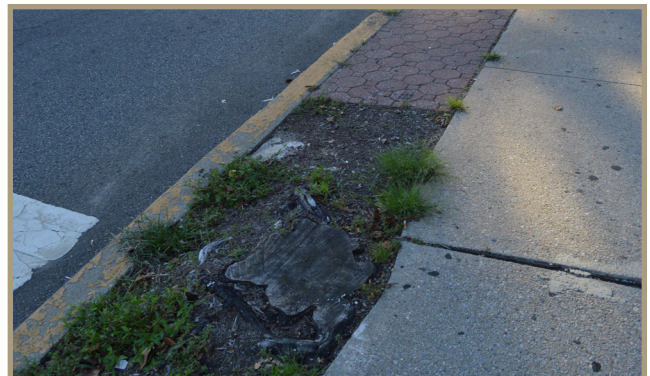
Figure 30. A tree that was not replaced, on Main Street.
