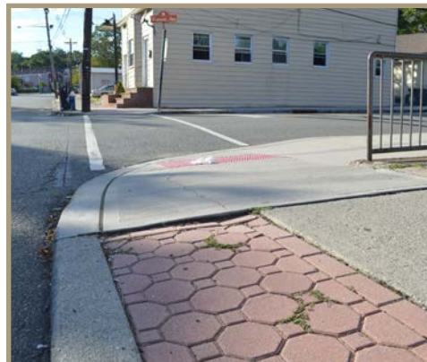
Figure 47. Looking north toward Watson Ave., an uneven transition could trip a pedestrian.
