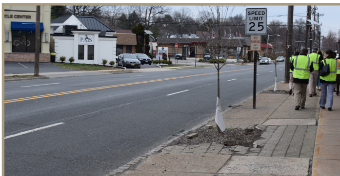
Figure 15. Cracked and uneven sidewalks and pavers, looking eastward on North Avenue near Central Avenue.
