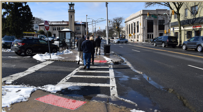
Figure 20. Misaligned accessibility ramp with drainage issues, looking westward at the train station entrance (photo taken during initial site visit).
