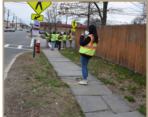
Figure 30. Cracked slate sidewalks near St. Paul Street, looking westward on North Avenue.
