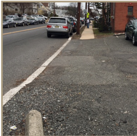
Figure 13. A sidewalk disappears in front of a parking lot along North Avenue, looking eastward on North Avenue. (Photo courtesy Lisa Lee, EZ Ride)
