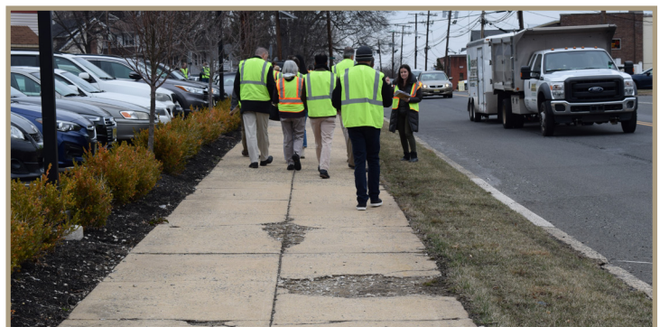
Figure 16. Crumbling sidewalk looking eastward on North Avenue near South Euclid Avenue.
