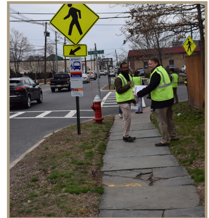
Figure 14. Cracked and raised slate sidewalks, looking westward at the intersection of St. Paul Street and North Avenue.
