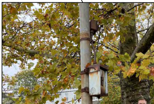
Unknown electrical service equipment
