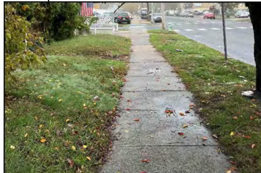
Overgrowth onto sidewalk limits use, ponding in some areas
