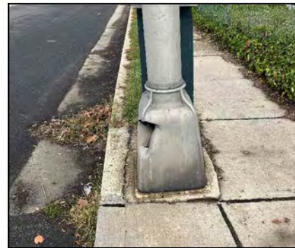
Damaged signal equipment
