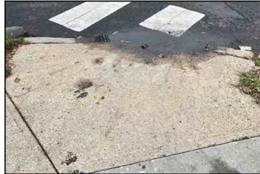
Curb ramp not ADA compliant, ponding observed
