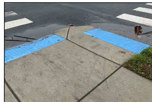
Ponding at curb ramps
