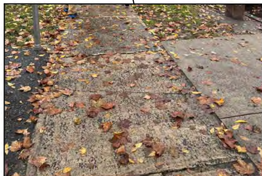
Sidewalk condition varies throughout corridor
