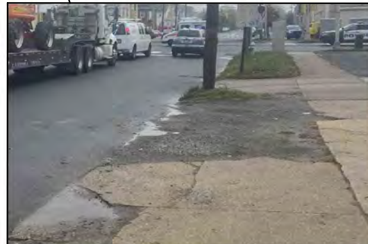
Many areas do not have curb
