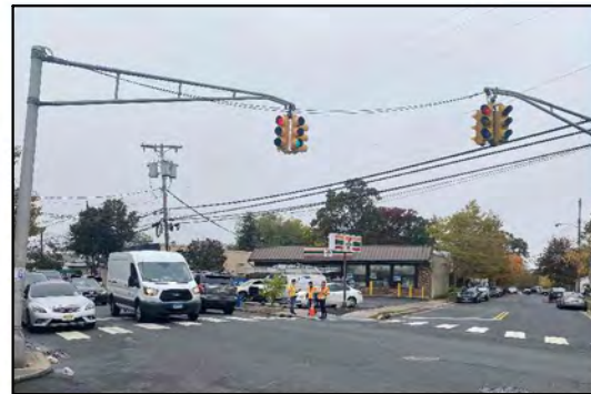
Outdated signal equipment, no pedestrian signal heads or push buttons
