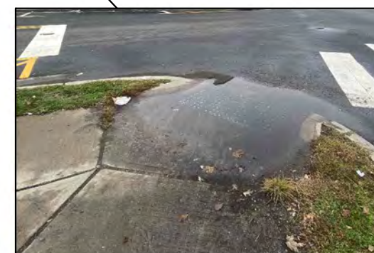
Ponding on curb ramp, can freeze in winter
