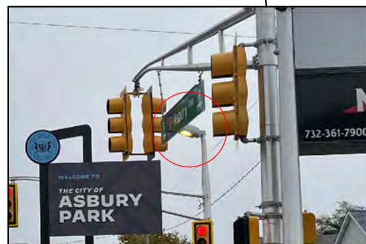
Mongoose light fixture on during daylight
