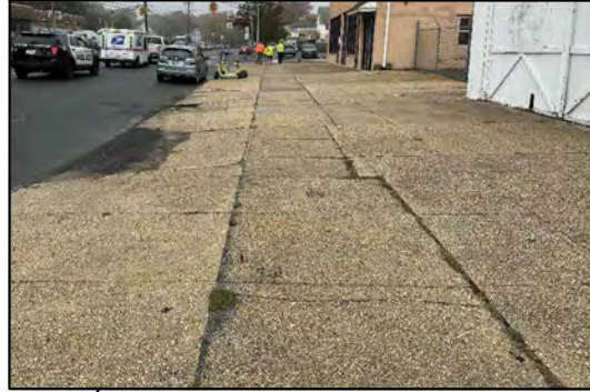
Wide concrete area may be confusing to road users
