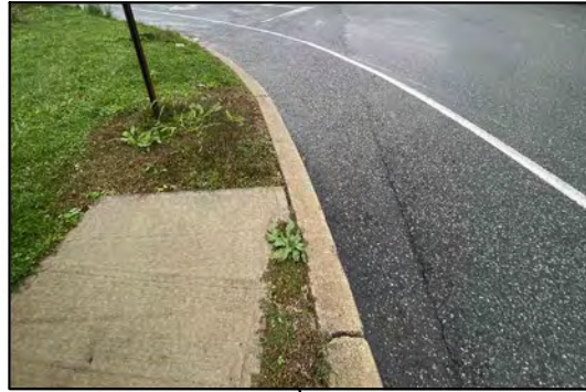
No curb ramp for sidewalk at intersection
