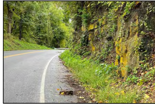
Rock face may obstruct sight distance
