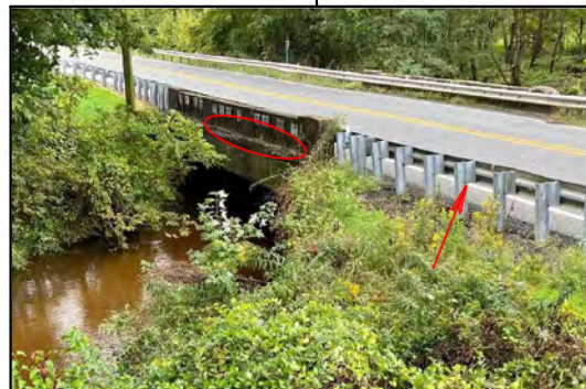
Guide rail does not meet current standards, missing concrete on structure
