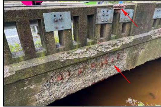
Missing concrete and exposed rebar on structure, guide rail does not meet current standards
