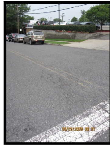
Faded yellow centerline
