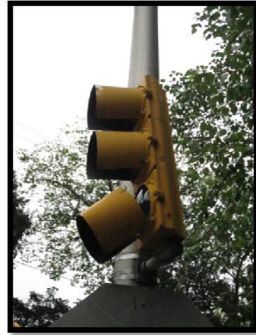
Traffic signal in disrepair
