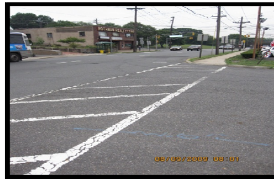
Partially faded crosswalk
