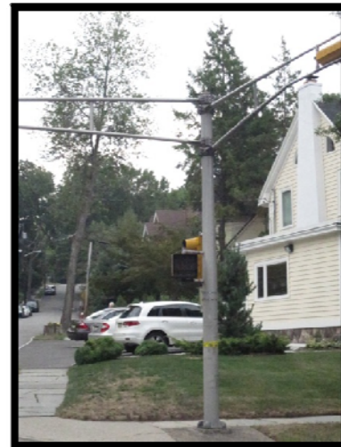
Pedestrian signal in disrepair
