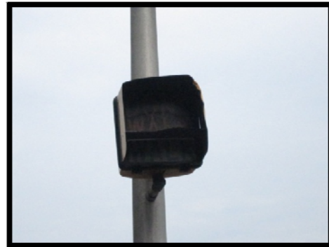
Pedestrian signal in disrepair
