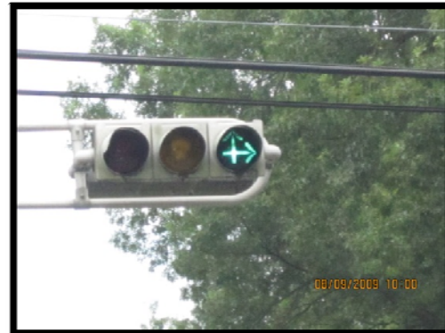
Traffic signals with arrows create conflict and are not standard.
