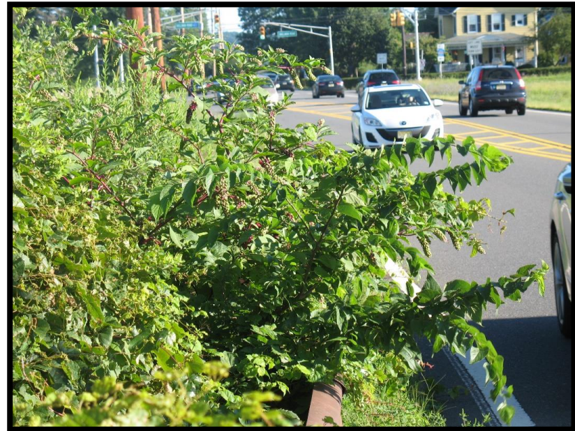
Vegetation needs to be trimmed
