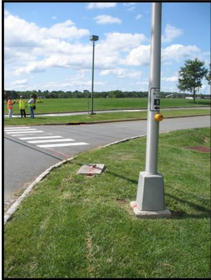
Lack of access to push button
