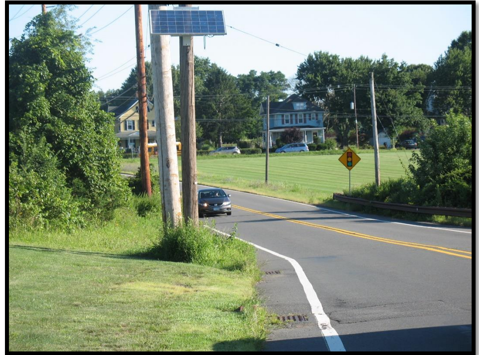
Vegetation and utility poles block sight distance
