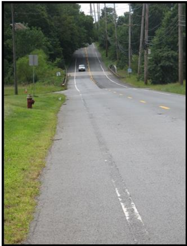
Worn pavement markings
