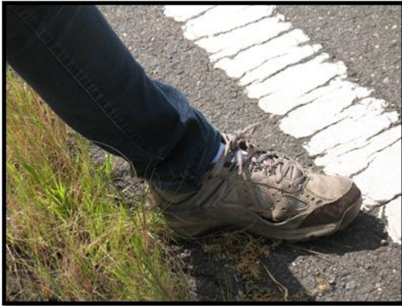
Lack of shoulder
