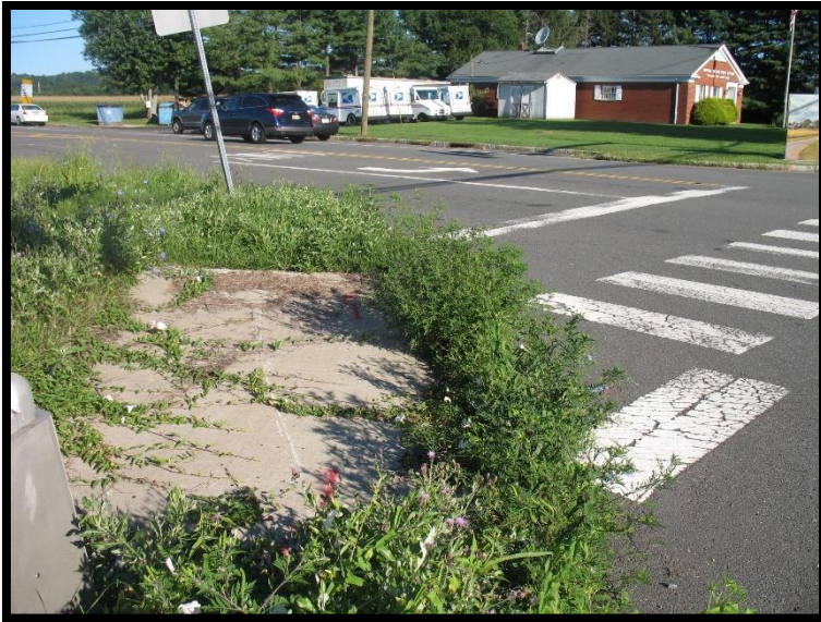
Lack of sidewalk connectivity
