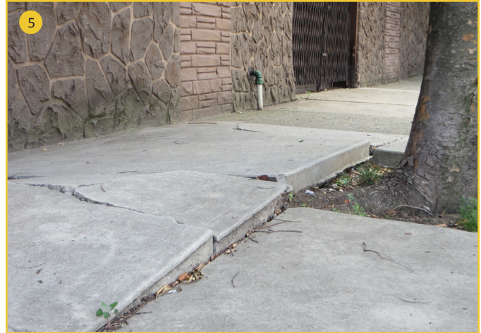
One example of uneven sidewalk
