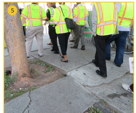
Uneven sidewalk surface
