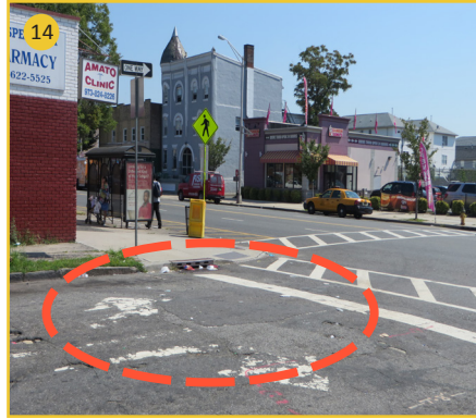
Faded pavement markings
