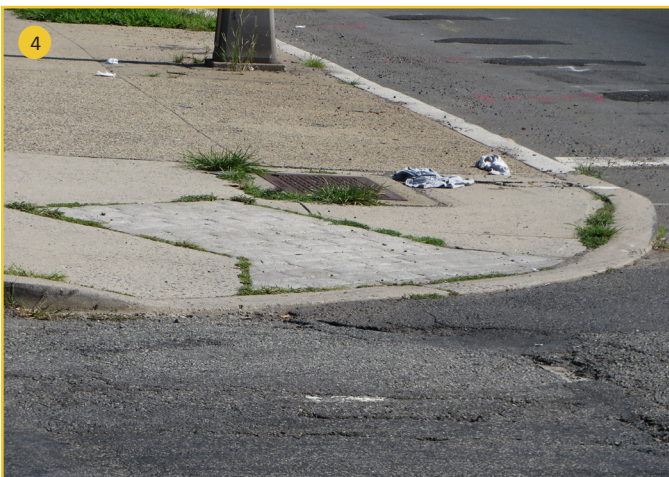
Curb ramps are not ADA compliant
