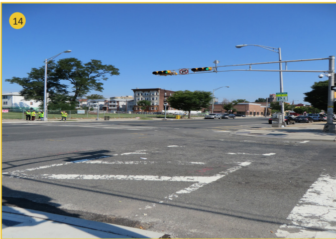
Faded pavement markings
