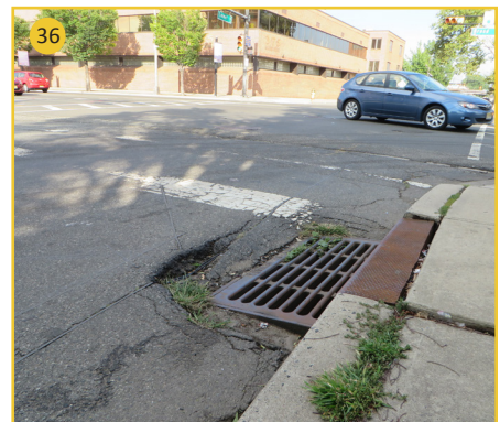
Depressed inlet and non-operational loops in pavement
