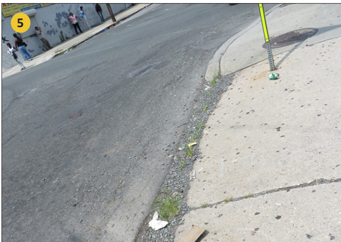
Unnecessary depressed curbs.
