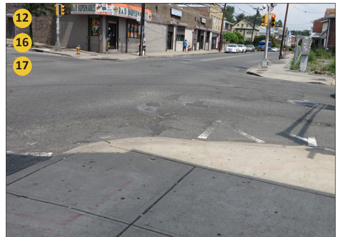
Faded crosswalks; Lack of truncated domes; No pedestrian signal heads.
