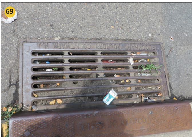
Drainage grate full of debris and is also not bicycle safe.
