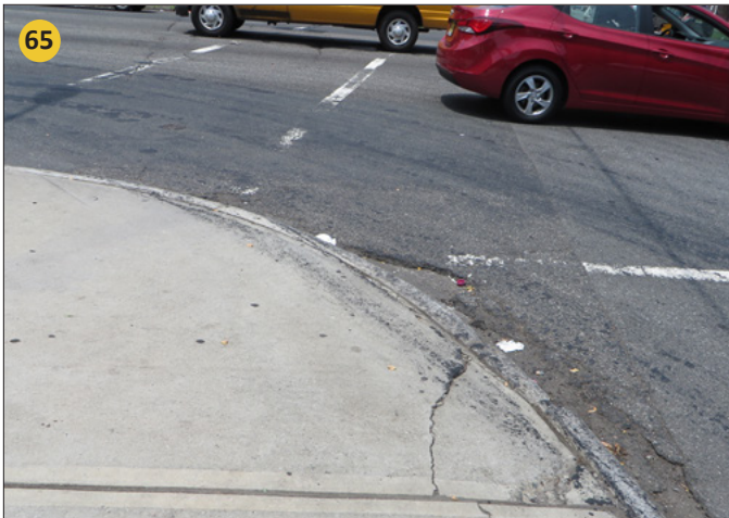
Missing curb cut on northeast corner and missing truncated domes on all corners.
