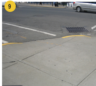
Faded crosswalks (above, #12), lack of tactile domes (right, #9).
