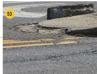
Deteriorated curb end.
