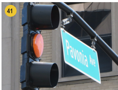
Missing visor on signal head.
