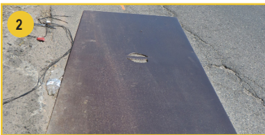
Metal plate in roadway
