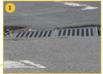
3 Sunken sewer grate.
