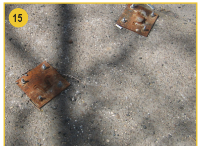
15 Metal plates (about 6" x 6") with screws sticking out on sidewalk.
