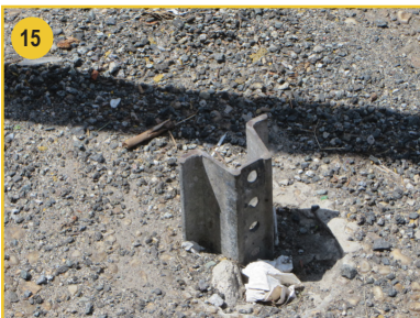
15 Abandoned breakaway post; Grit (presumably from the road) on sidewalk.
