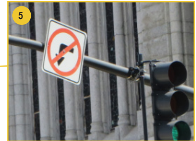
"NO LEFT TURN" sign is skewed downwards.
