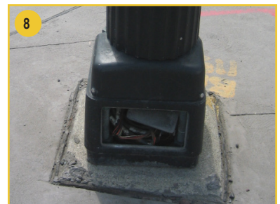
Foundation missing plate on southwest corner.
