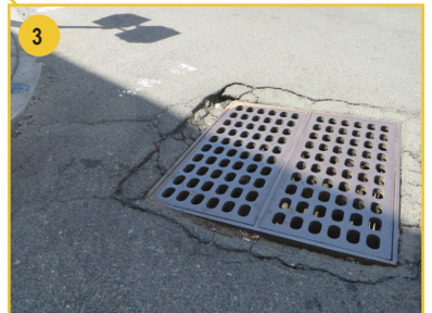
3 Sunken grate needing maintenance.
