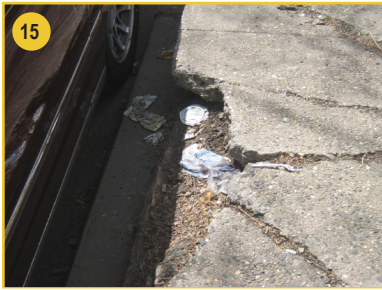
Broken sidewalk pavement.
