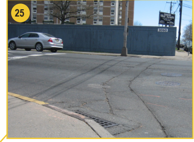
25 Missing crosswalk on north leg. Also missing "USE OTHER CROSSWALK" pedestrian signage.
