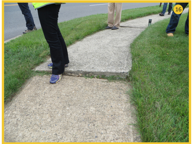
Figure 33 – Sidewalks are in poor condition
