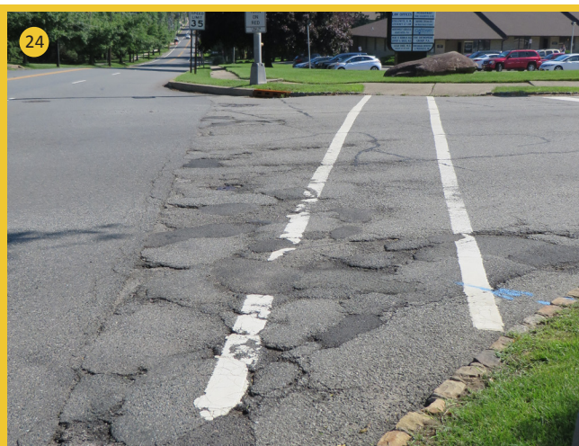
Figure 35 – Pavement and markings in poor condition
