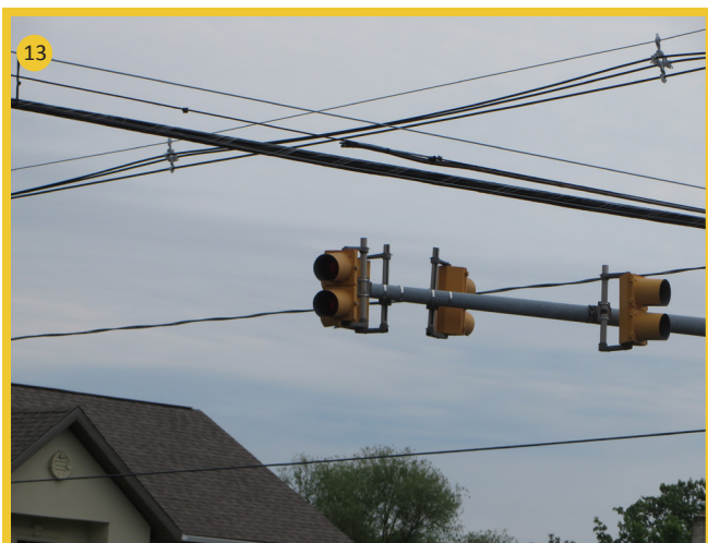
Figure 40 – Flashers are small and not clearly visible
