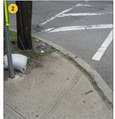
Lack of curb cut at Lexington Street
