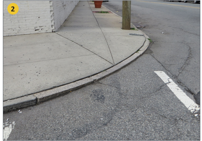
Lack of truncated domes
