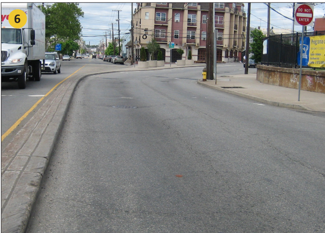
Faded pavement markings
