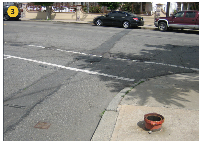
Tripping hazard in sidewalk; lack of marked crosswalks or signals to cross Ferry Street; parking in intersection which limits visibility of pedestrians in crosswalk
