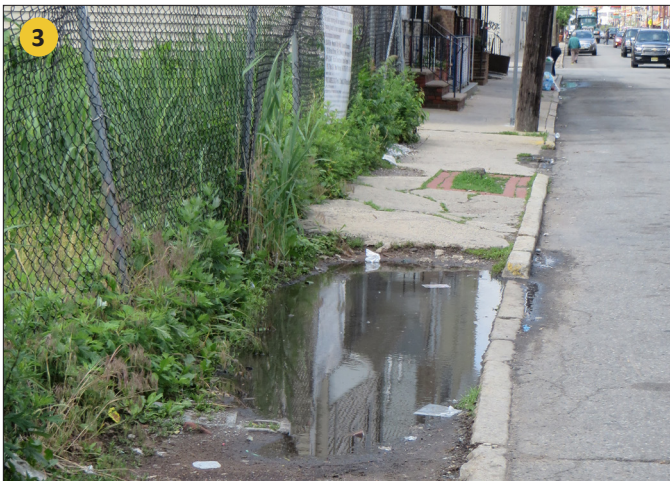
Portions of the sidewalk are flooded, rendering them unusable.
