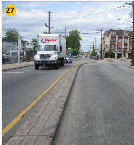
Median is too narrow and inadequately demarcated; stop bar is severely faded
