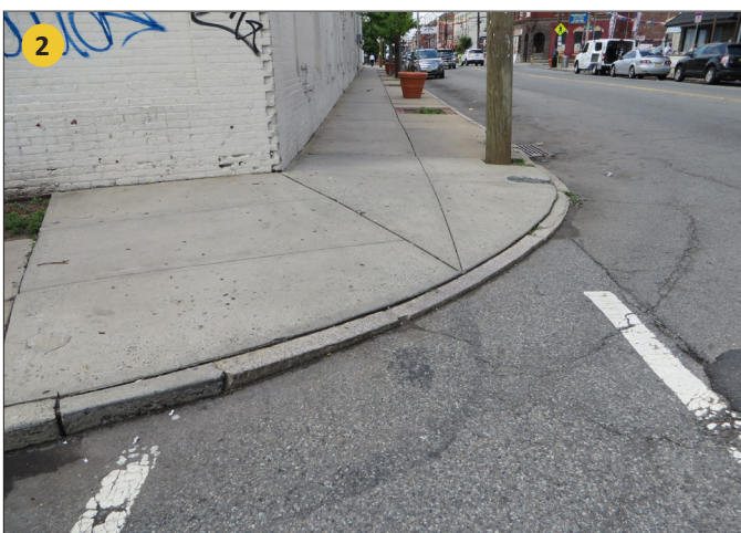
The intersections lacked true ADA facilities (e.g. tactile pads and curb cuts).
