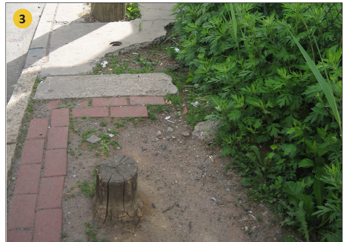
Tripping hazards in sidewalk
