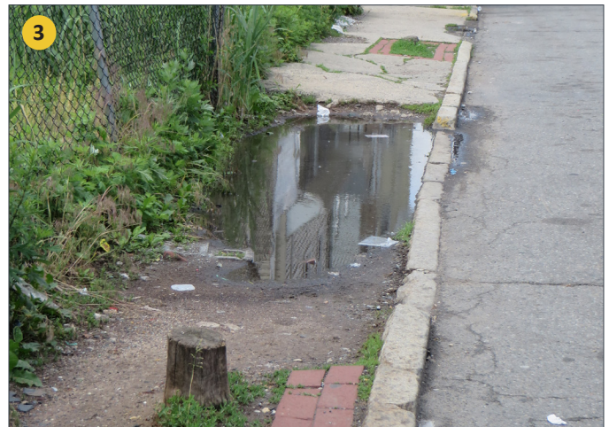
Pooling and tripping hazards in sidewalk
