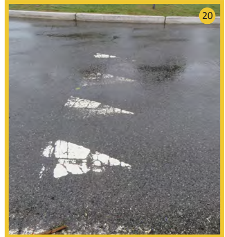
Faded pavement markings
