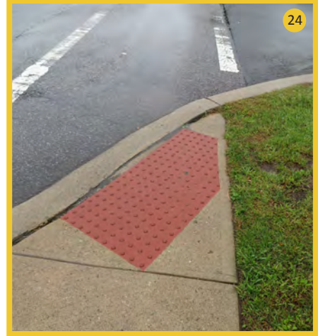
ADA facilities are not fully ADA compliant
