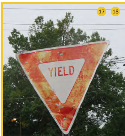
Signs in poor condition
