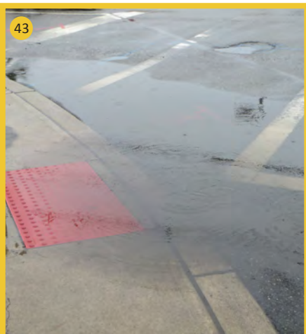
Ponding issue at southeast corner
