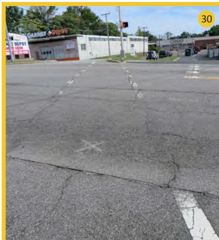
Pavement markings are faded
