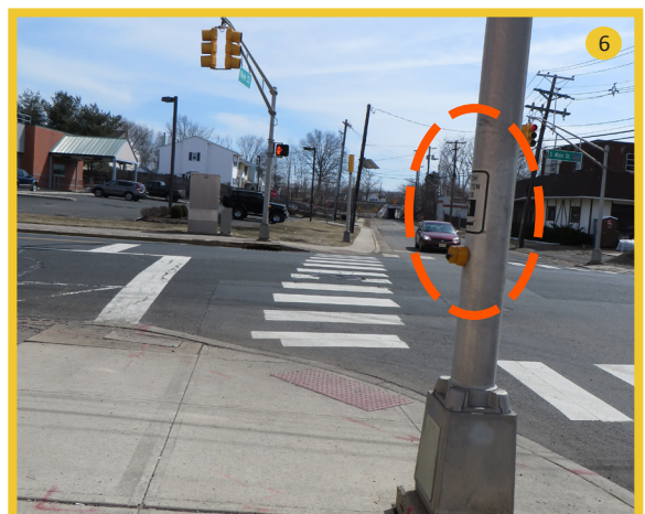
Pedestrian push button not located near the crosswalk
