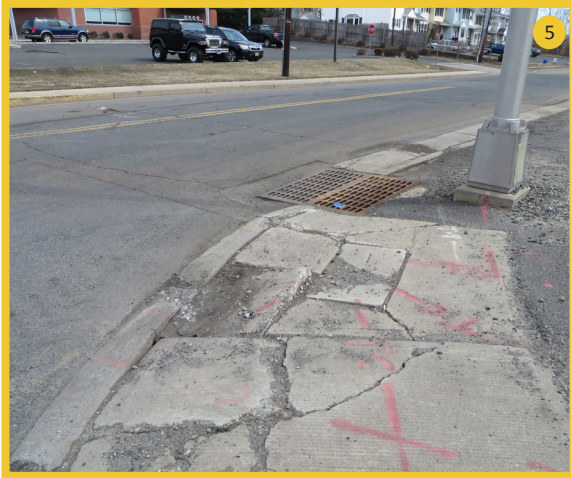
ADA facilities are lacking
