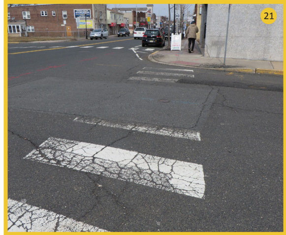
Faded pavement markings
