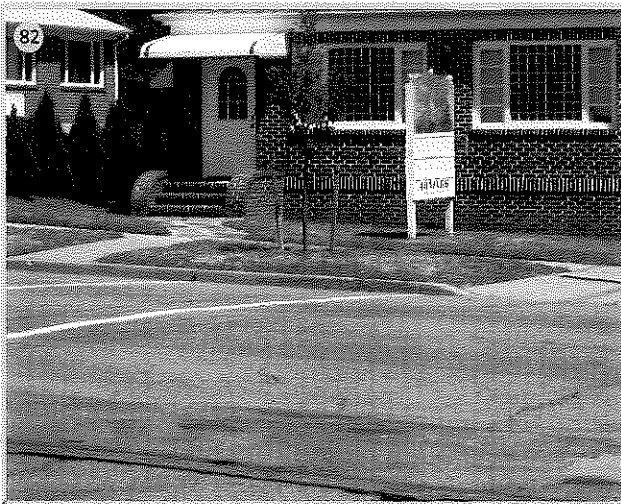
There is no depressed curb or ramp at end of crosswalk
