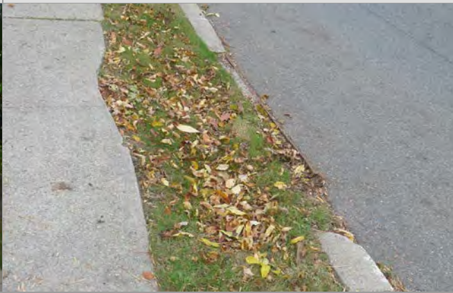
Missing section of curb
