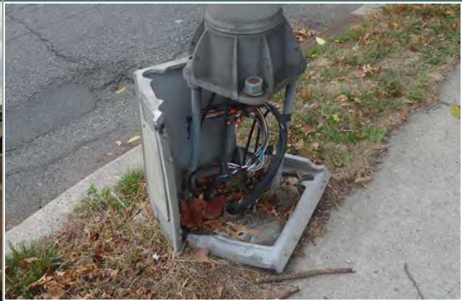
Broken traffic signal transformer base
