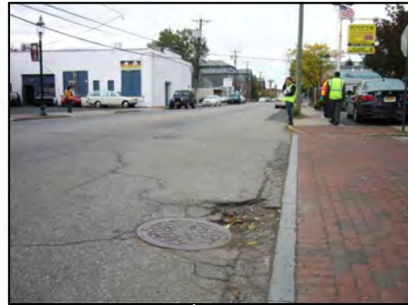
Pavement cracks within the intersection and along curblines
