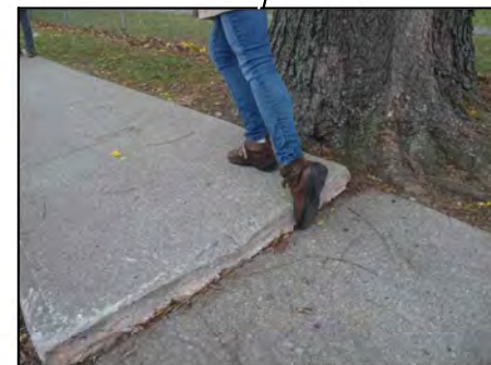
Sidewalks are in poor condition and can be a tripping hazard
