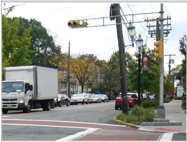
Signals lack pedestrian signal heads
