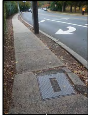
Sidewalks are not ADA compliant
