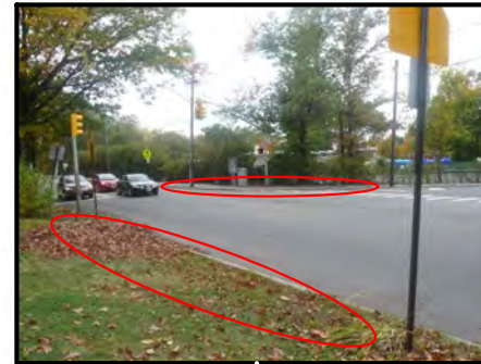
Wide curb radius in SW corner; Missing sidewalk on East side
