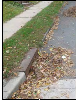
Poor drainage conditions on many roadside inlets
