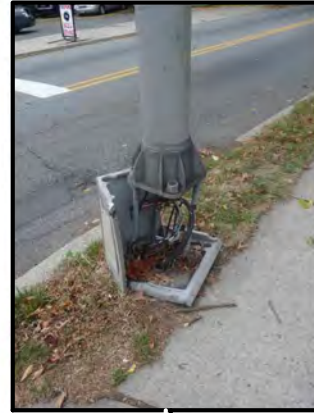
Broken traffic signal foundation, the foundation is not breakaway
