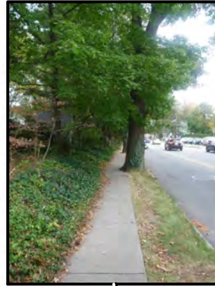
Curb cuts to accommodate trees; not ADA compliant
