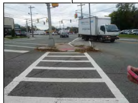
Pedestrian island is too small with no room for a landing area
