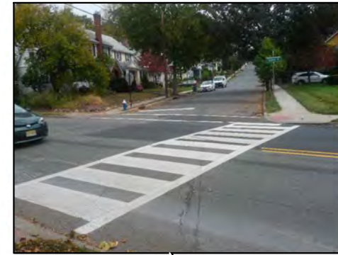
There is no pedestrian signage at or around pedestrian crosswalk
