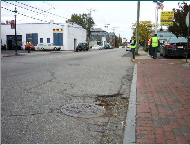
Edge of roadway pavement is inadequate for bicyclists
