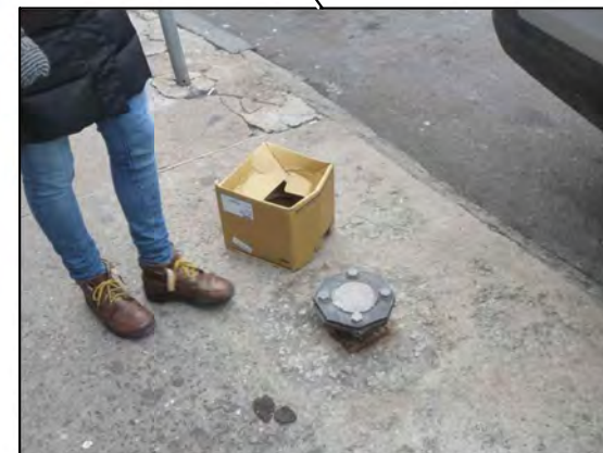
Tripping hazard within sidewalk.
