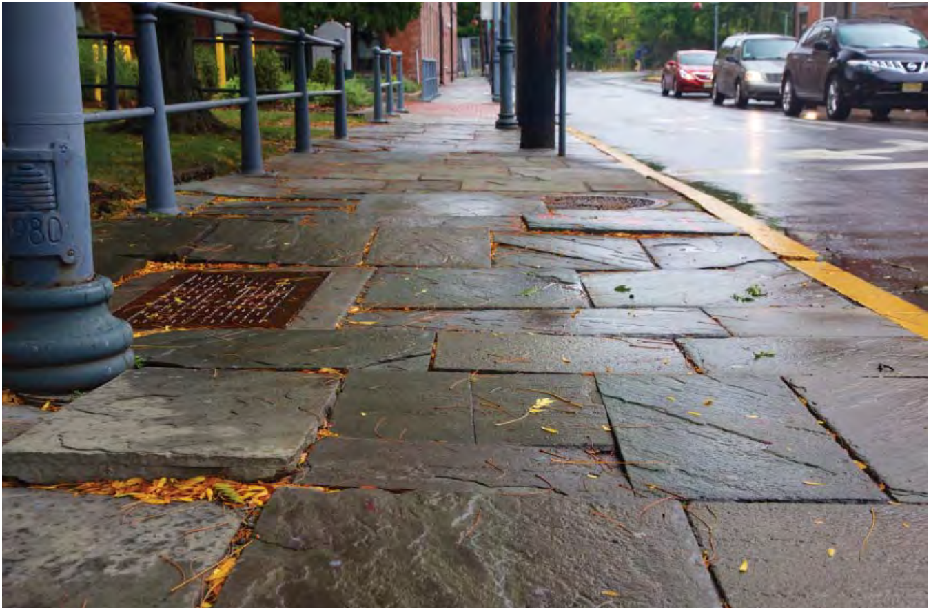
Potentially challenging sidewalks for wheelchairs and walkers alike
