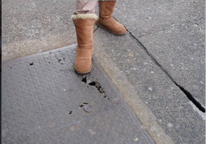
Underground vaults exist under sidewalks; cellar doors are rusted, and sidewalks have cracks
