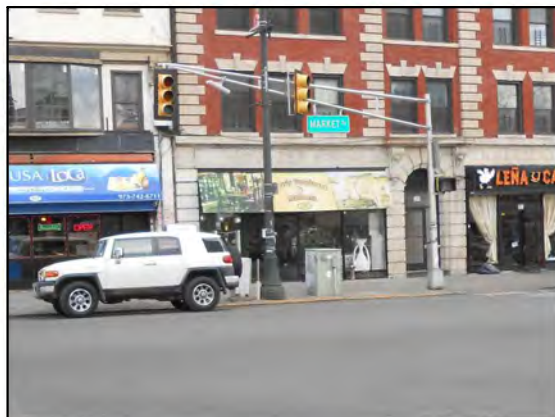
The signal poles and heads are installed, but are not operational.
