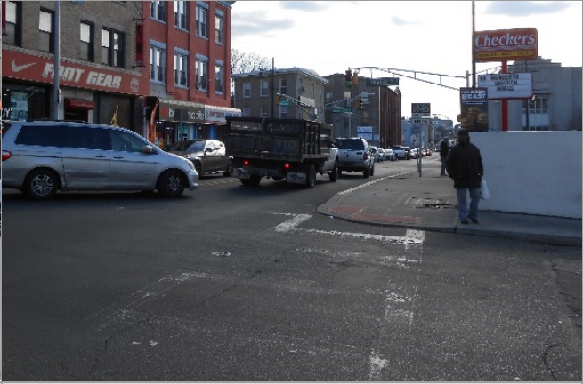
Many crosswalks need restriping
