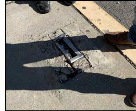
Portion of traffic signalpole foundation not removed; could pose tripping hazard
