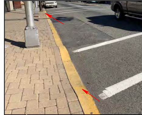
No detectable warning surfaces on paver curb ramps
