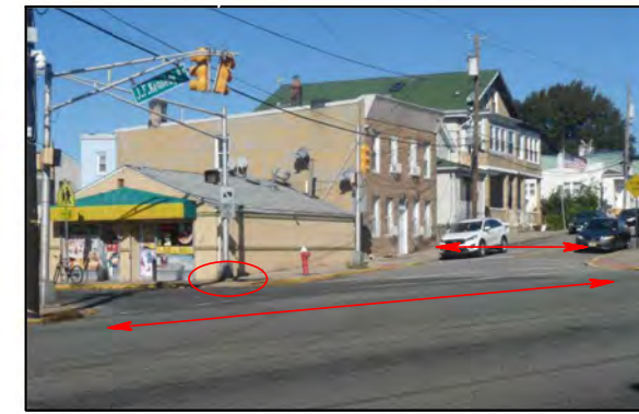
Long crosswalk with worn striping and one curb ramp that does not align to any marked crossing may be confusing to road users (Similar intersection has different marked crosswalk locations)
