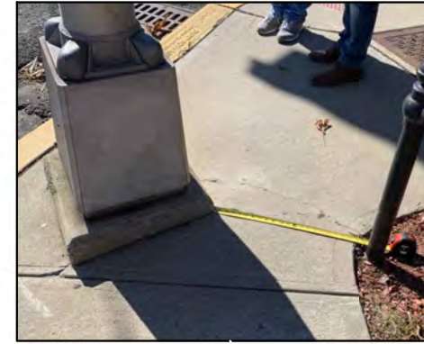
Insufficient clear width for ADA compliance
