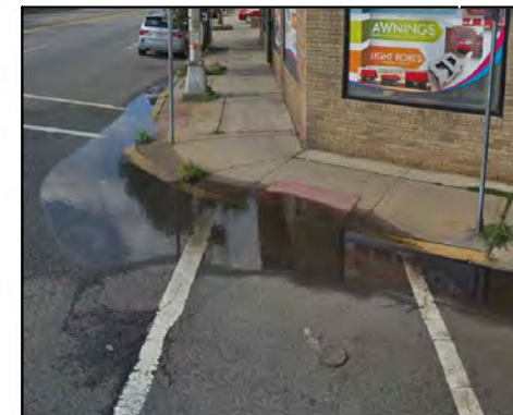
Standing water at curb ramp and edge of road, which can freeze in cold conditions, and create a hazard for pedestrians
