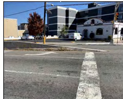
Median barrier lacks current impact attenuators
