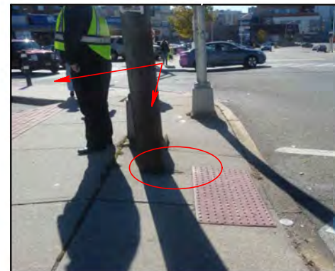
Foreground: Utility pole within curb ramp Background: Crosswalk may not follow pedestrian path
