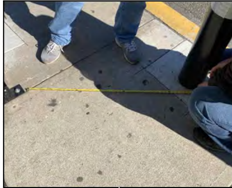
Bollards encumber pedestrian path around bus shelter (clear area less than 4' wide)
