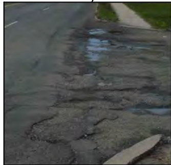
Poor pavement condition
