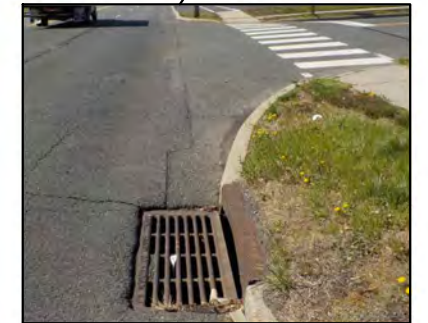
No ADA ramps or bicycle safe grates
