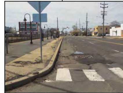
Incorrect cross slope along train station curb
