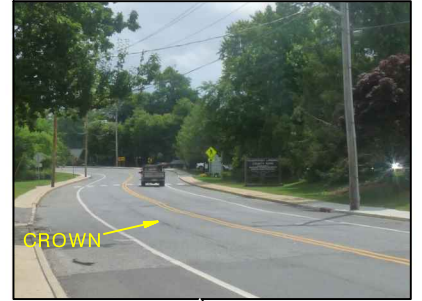
Pedestrian crossing infrequently used with no ADA ramps. Roadway crown in EB lane (i.e. not along center line)
