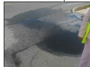
Ponding observed at intersection corners and curb ramps
