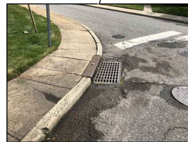
Sidewalks and pavement in poor condition; inlets filled with water; no ADA curb ramps
