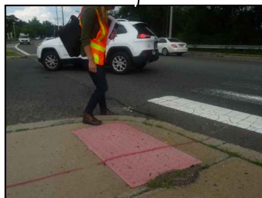
No ADA compliant curb ramps; faded crosswalk
