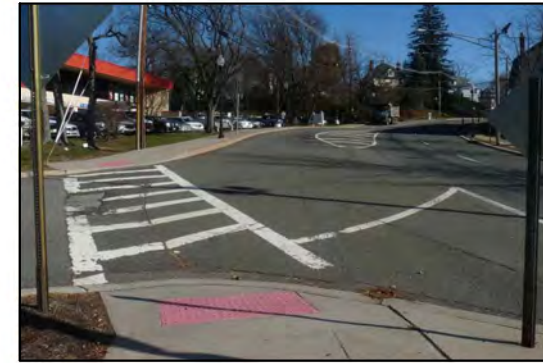
Roadway alignment limits visibility of and for pedestrians; wide pavement may promote speeding
