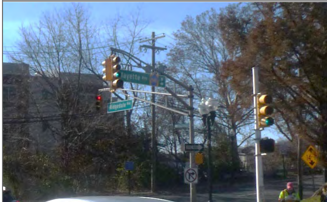
9. Signal heads can be upgraded to 12" with backplates for better visibility
