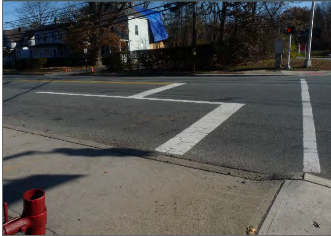
7. Lane use not clearly defined
