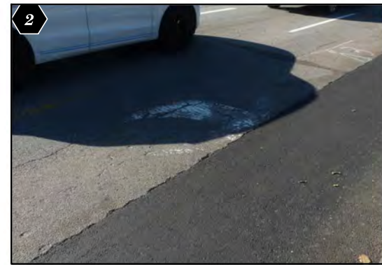
Worn pavement markings do not alert drivers to exclusive lane use
