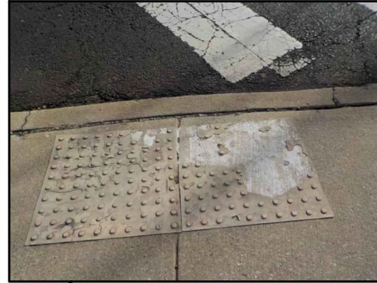
Detectable warning surfaces not contrasting color and are in poor condition
