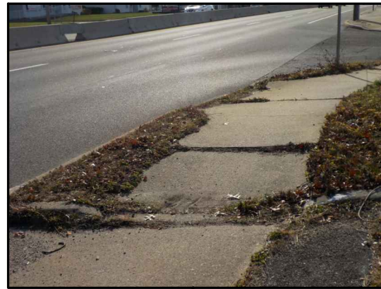
Uneven/damaged sidewalk can be a tripping hazard
