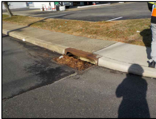
Inlet filled with debris presents drainage issue
