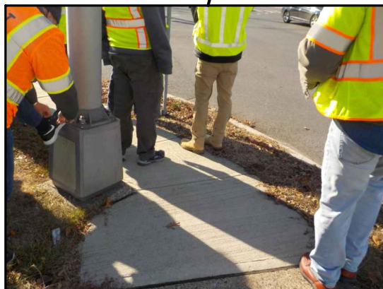
Protruding signal foundation in sidewalk can be a tripping hazard
