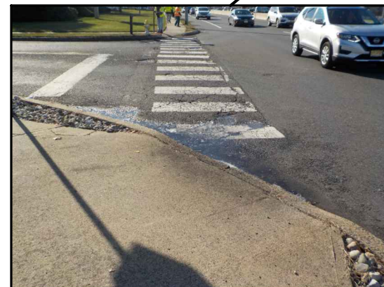
Ponding at curb ramps; non-compliant ADA ramps
