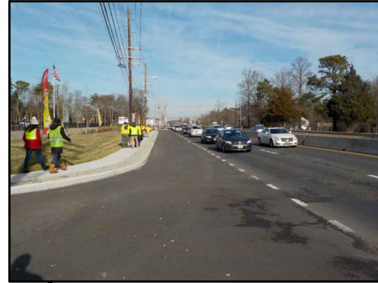
Pavement markings to indicate right turn only are missing
