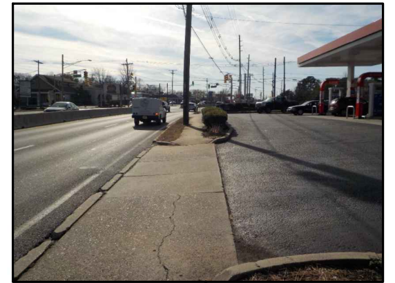
Wide driveways close to intersection creates access management issues
