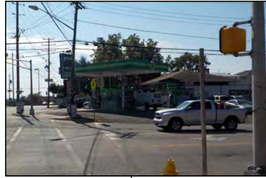
Pedestrian signal heads not on both sides of crossing at intersection
