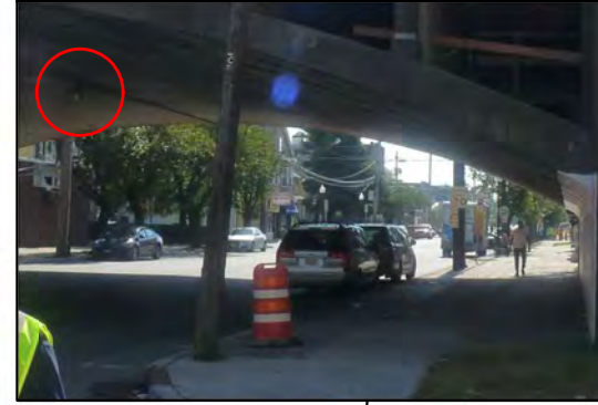
Lighting under structure may be insufficient at night
