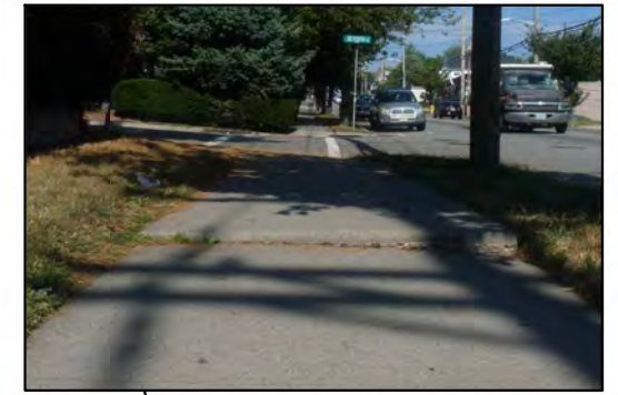
Uneven sidewalk is a tripping hazard
