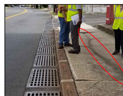
Collapsed/uneven sidewalk above inlets can be a tripping hazard
