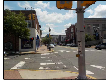
Non-compliant ADA ramps and worn crosswalk striping
