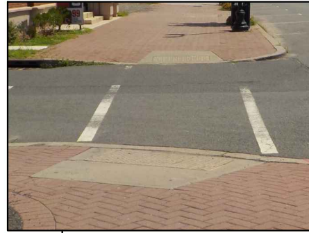
Detectable warning surfaces not contrasting color; worn crosswalk striping
