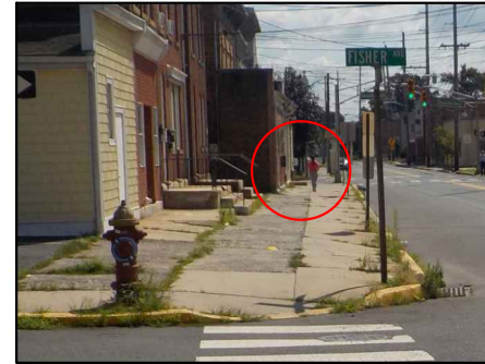
Uneven/damaged varying width sidewalk; steps protrude out; lacks ADA ramps
