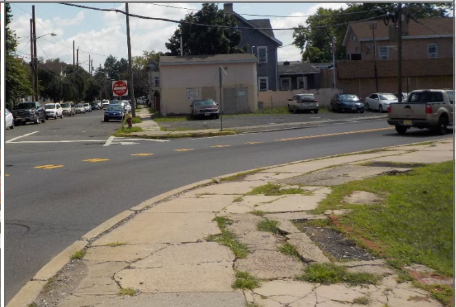
12. Sidewalk in poor condition
