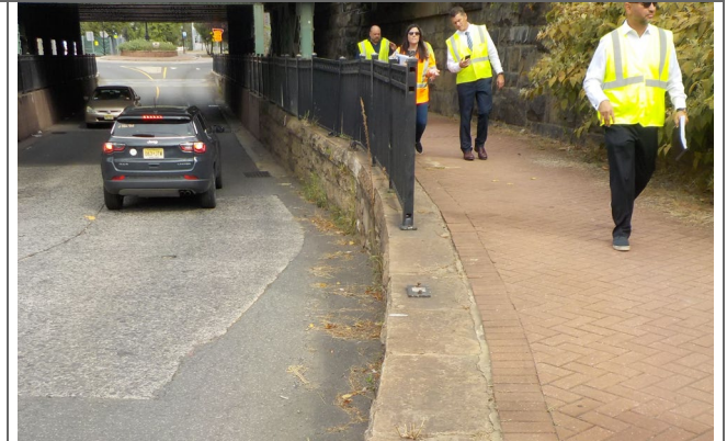
10. Fence needs replacement (along South Main Street)
