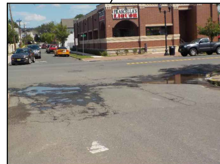
Ponding at numerous curb ramps
