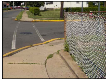
Lack of ADA ramps, worn striping and fence blocking visibility
