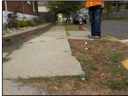
Broken/uneven sidewalk in NW corner of North St; lacks ADA ramps
