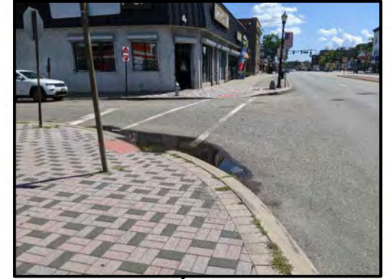
Ponding at curb ramp
