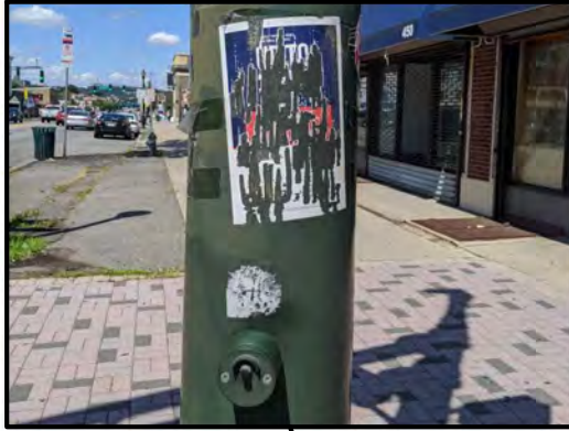
Pedestrian push button missing associated crossing sign
