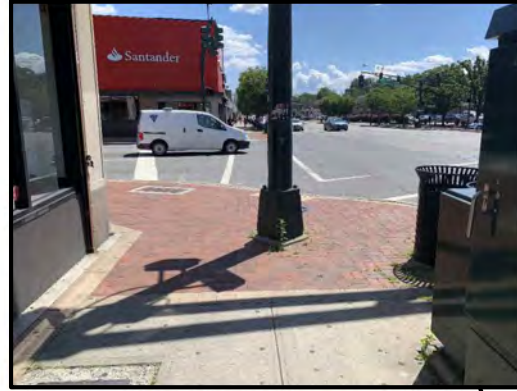
Traffic signal pole blocks pedestrian access route
