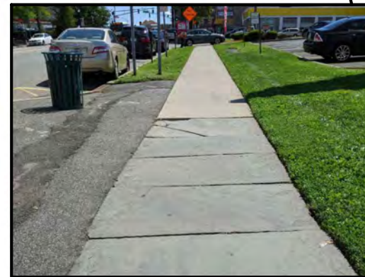
Inconsistent sidewalk material
