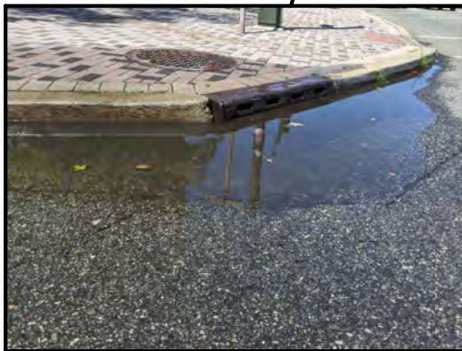
Ponding at inlet, needs to be cleared of debris
