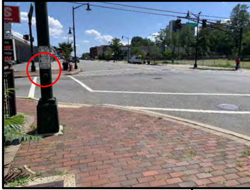
Pedestrian push button installed on incorrect side of traffic signal pole
