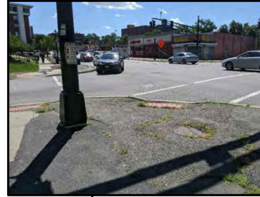
Sidewalk in poor condition, utilities located within curb ramp
