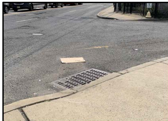
Curb ramps not ADA compliant Inlet in ramp travelway
