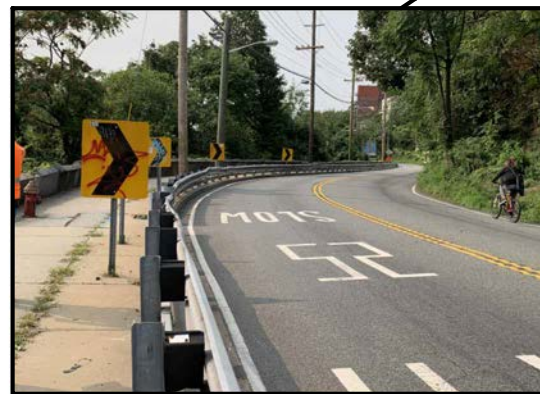
Damaged guide rail and defaced signs Limited sight distance along roadway
