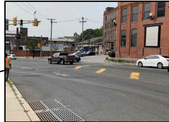
Wide pavement section with worn striping
