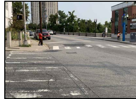
Non-compliant curb ramps and worn striping
