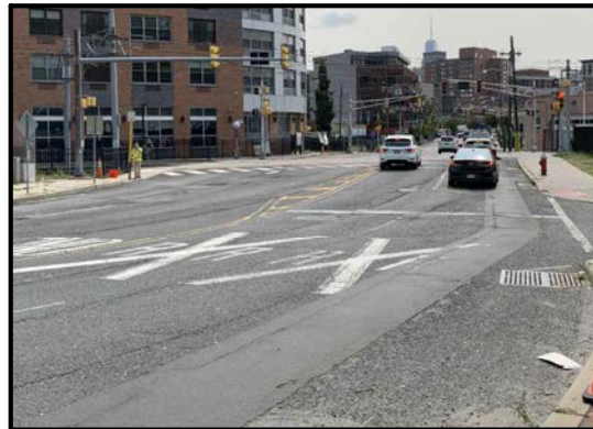
Pavement and markings in poor condition
