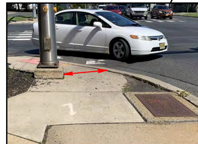
Passing space between pole and curbline may be insufficient
