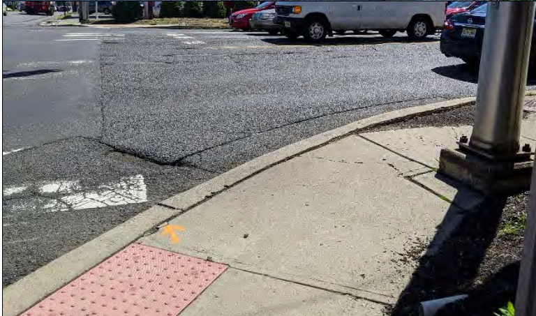
Pavement and sidewalk conditions vary. Newman Springs Rd at Shrewsbury Ave
