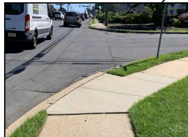
Curb ramps not ADA compliant
