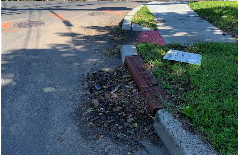
Debris covering curb ramp and inlet. Newman Springs Rd at Springdale Ave
