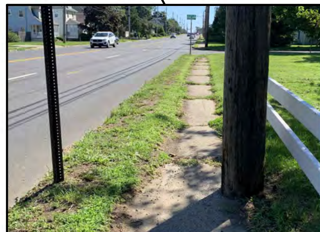
Sidewalk in poor condition and passing space restricted by utility pole and vegetation
