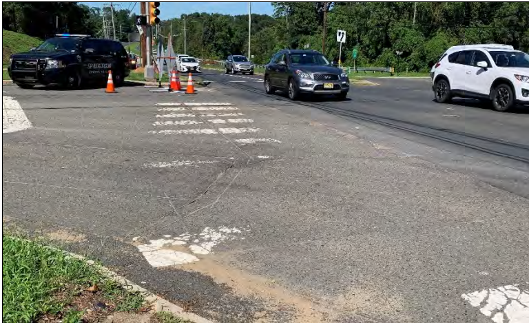
Worn crosswalk striping. Newman Springs Rd at Hance Ave
