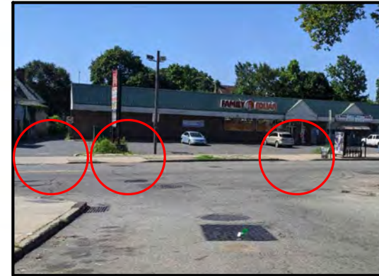
Multiple curb cuts with ramps not clearly defined or ADA compliant
