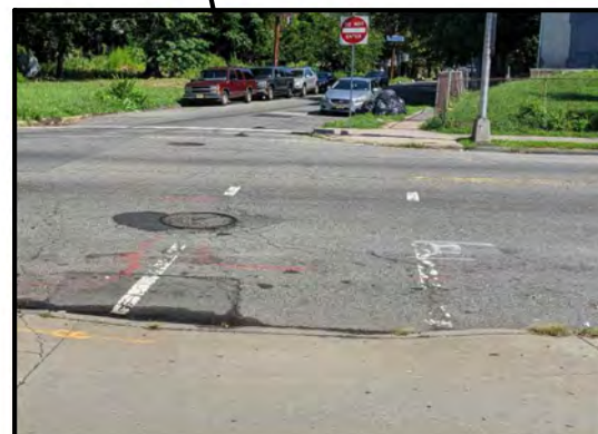
Ramps not ADA compliant Crosswalk striping worn
