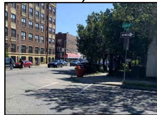
Curb ramps not ADA compliant Striping worn
