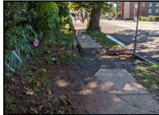
Damaged/ missing sidewalk may pose a tripping hazard; vegetation overgrown
