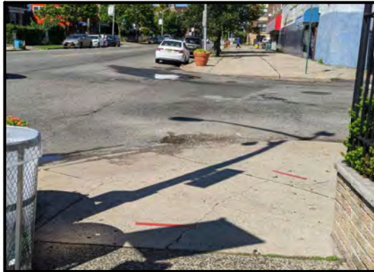
Ramps not ADA compliant Vehicle parked too close to corner
