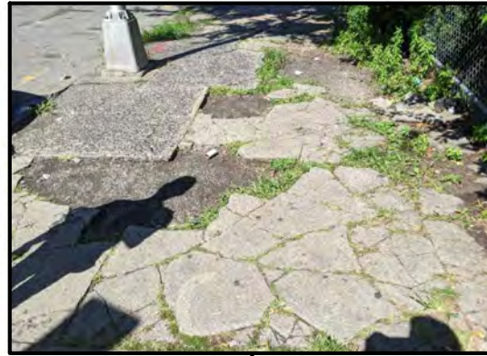
Damaged/ missing sidewalk may pose a tripping hazard
