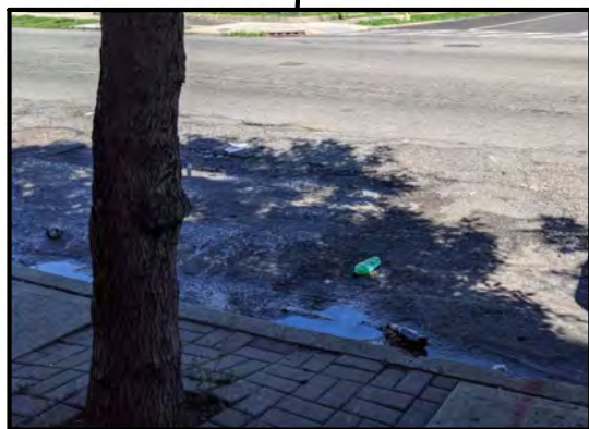
Area susceptible to flooding Ponding along roadway
