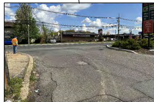
No marked crosswalk, no ADA curb ramps Missing stop bar and stop sign
