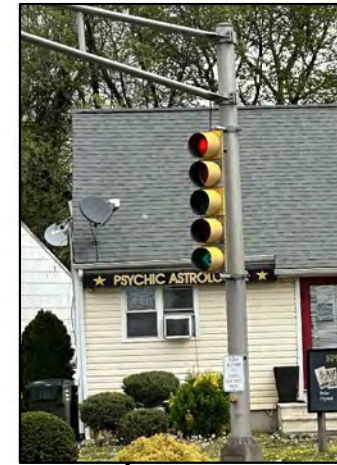
Outdated pedestrian push buttons and sign; No pedestrian signal heads
