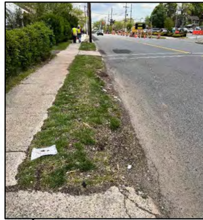
Missing curb along sidewalk
