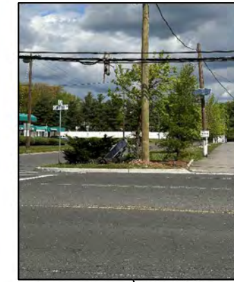
No marked crosswalk, ADA curb ramps and sidewalk; Remnant utility debris; Lack of lighting
