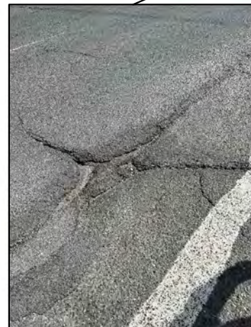
Poor pavement condition
