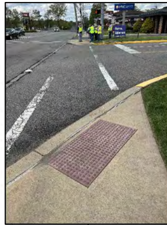
Faded crosswalk markings
