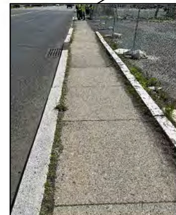
Missing edge lines and shoulder lines; tripping hazard due to uneven sidewalk; no offset between sidewalk and roadway
