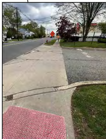
Poor condition along walkway
