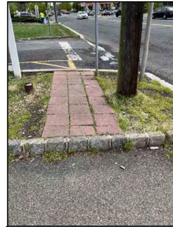
Missing ADA curb ramps, missing sidewalk
