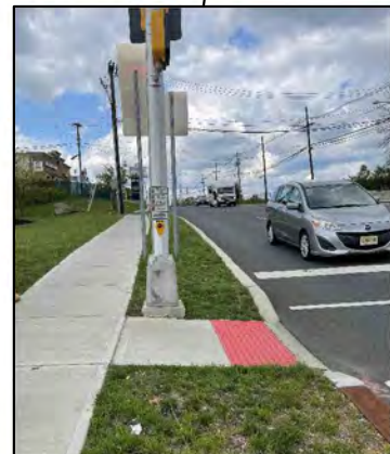
Steep ADA curb ramp cross slope; Missing ADA curb ramp flares
