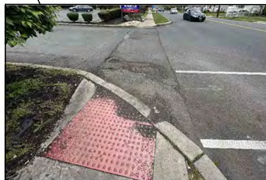
Non compliant ADA curb ramps; Missing crosswalk
