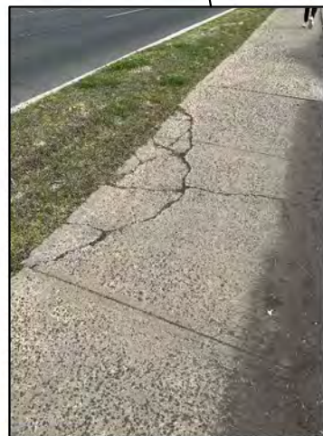
Poor sidewalk condition
