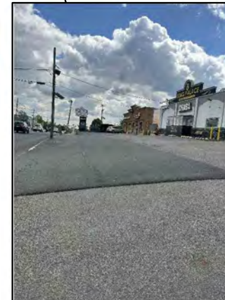
Steep slope across driveway and lack of concrete sidewalk
