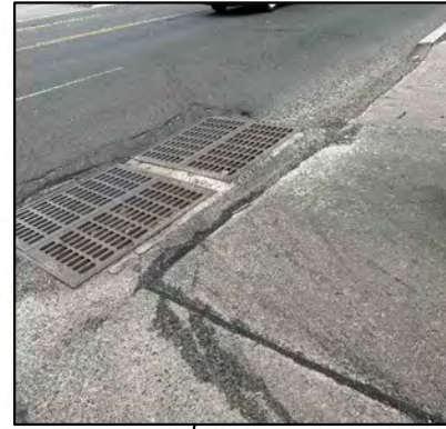
Poor pavement condition near inlet
