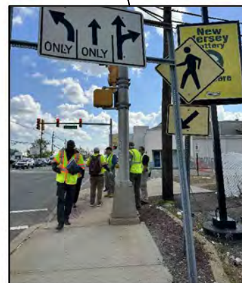
Pedestrian crossing sign at incorrect location; Low vertical clearance for lane usage sign
