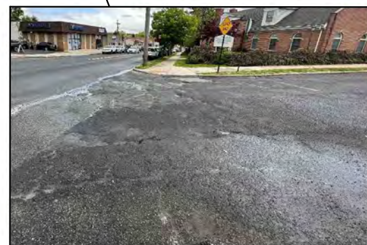
Poor pavement condition; Faded stop bar marking
