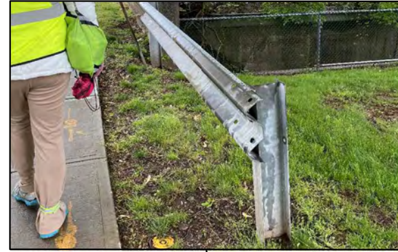
Guide rail not compliant
