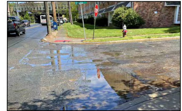
No marked crosswalk and drainage issues along crosswalk; Faded stop bar marking; Bent sign posts; Stop sign height clearance inadequate
