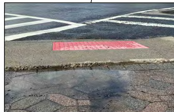
ADA curb ramp and adjoining paver sidewalk results in uneven pedestrian path
