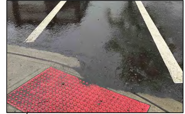
Ponding / Drainage issues at ADA curb ramps
