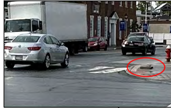
Foundation tripping hazard in sidewalk; Faded crosswalk
