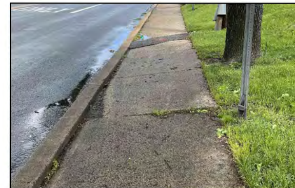
Steep sidewalk slope
