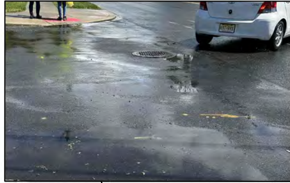
No marked crosswalk; Drainage issues along crosswalk
