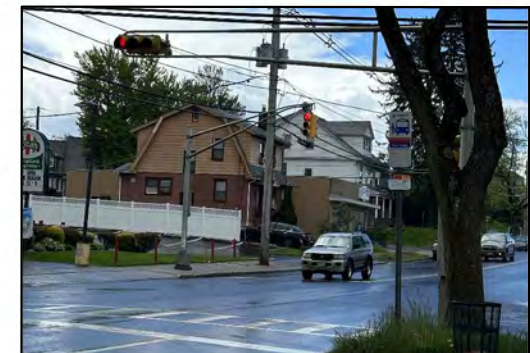
Outdated traffic signal; Missing pedestrian signal equipment
