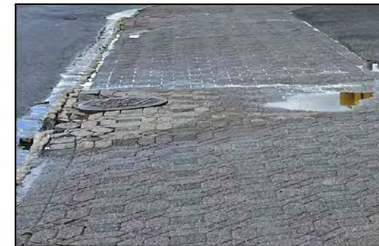
Drainage issues along sidewalk; Dips in curb
