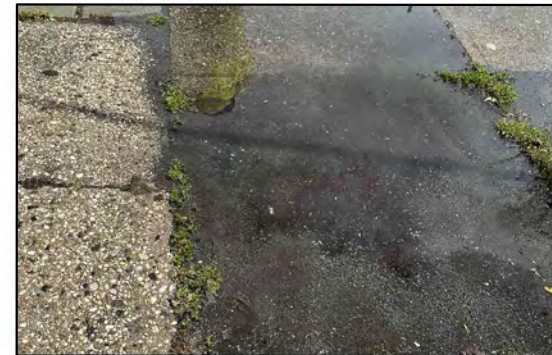
Drainage issues along sidewalk
