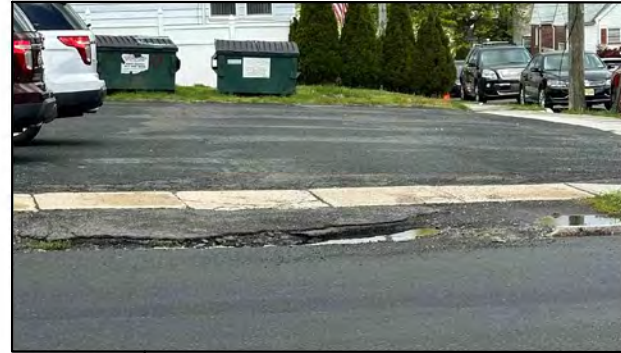
Driveway in poor condition
