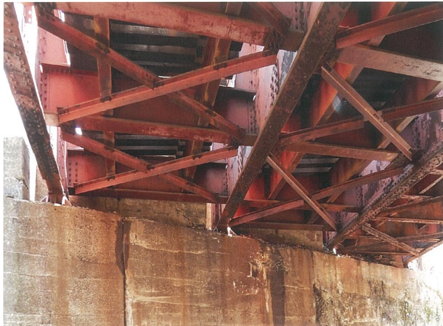
PHOTO 5-6: General view of the superstructure, looking east. Note paint peeling with corrosion throughout the superstructure steel.
