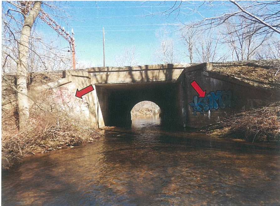
PHOTO 5-1: South elevation, looking north. Note tree growth in front of the southwest wingwall and graffiti (arrows) at the southeast and southwest wingwalls.
