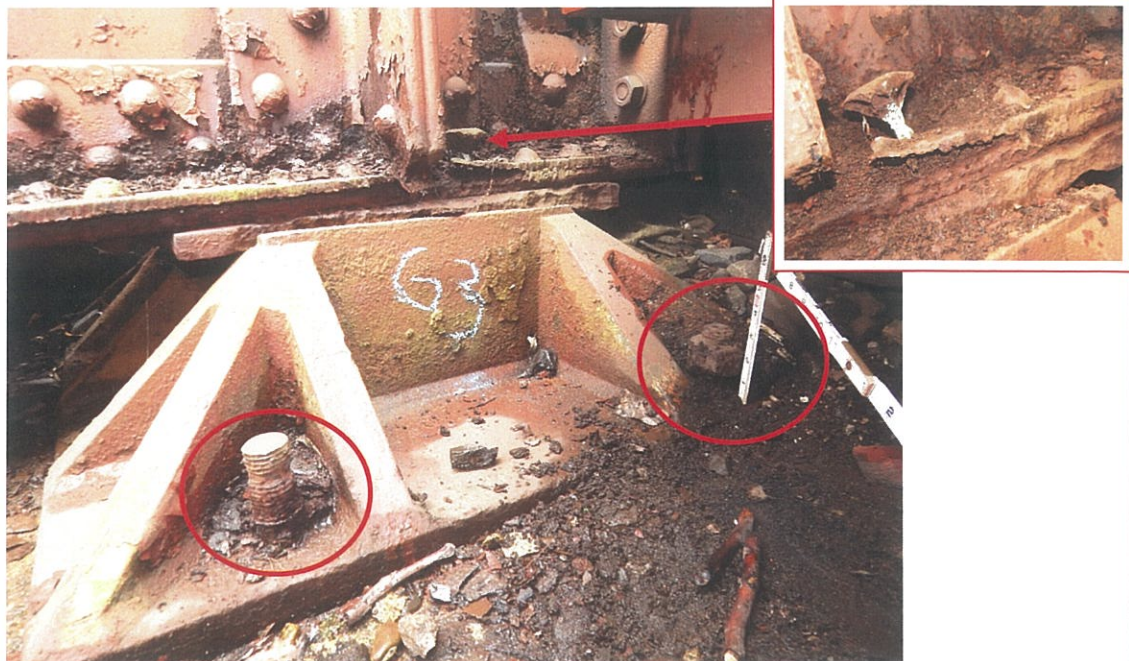
PHOTO 5-16: Missing and raised anchor bolt nuts (Circles) at the north side of Girder G3 bearing over the west abutment, looking southwest. Note up to 100% section loss to the sole plate bolt (Insert). Note also, the bearing is seized.
