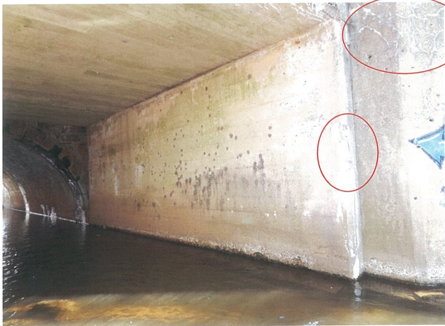
PHOTO 5-8: General view of the east abutment breastwall of concrete slab, looking northeast. Note fine cracks with efflorescence at top of the southeast wingwall. Note also, small spall with heavy efflorescence along the south edge, approximately located at mid height of the breastwall.
