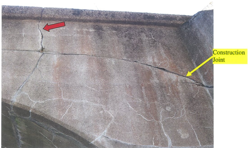
PHOTO 5-10: Wide crack at west end of the north spandrel wall, looking south (arrow). Note fine map cracks with efflorescence.
