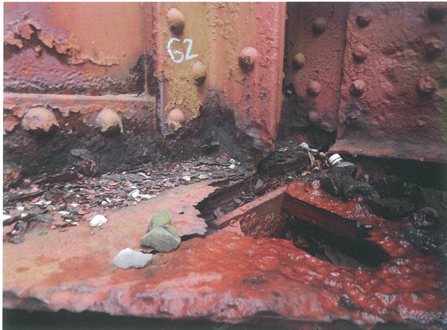
PHOTO 5-15: Severe section loss and holed through gusset plate at the south side of Girder G2 bearing over the east abutment, looking northeast.
