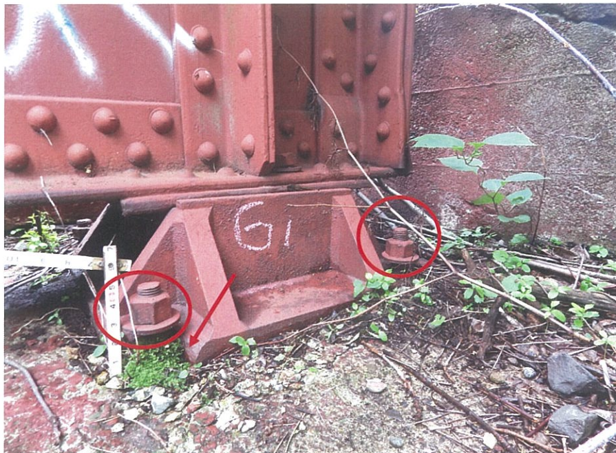
PHOTO 5-8: General view of bearing G1 over the east abutment, looking northeast. Note raised anchor bolt nuts (Circles) and broken masonry plate at the southwest corner of the bearing (Arrow).
