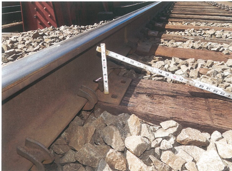
PHOTO 5-12: Raised spike at the south rail on Track #1 at the east approach, looking southwest.
