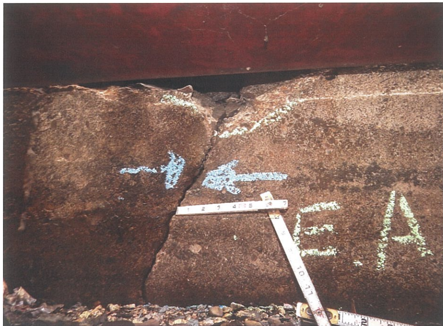
PHOTO 5-20: 1/4" wide crack and small spall at the east abutment backwall between Girders G3 and G4, looking east.
