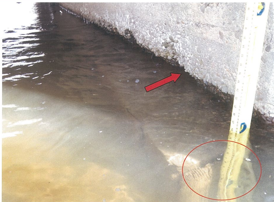
PHOTO 5-11: Moderate to severe scaling along the bottom of east abutment breastwall of concrete deck slab, looking northeast. Note exposed footing at south end (typical throughout the length of the breastwall).
