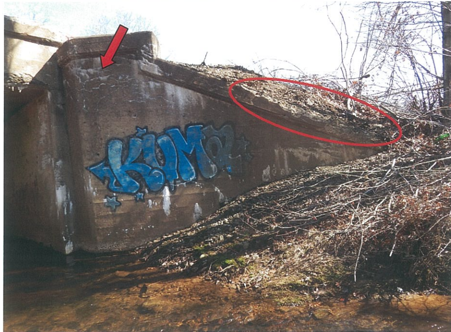
PHOTO 5-13: Large spall (circle) along the top face of the southeast wingwall, looking northeast. Note scattered fine cracks with efflorescence (arrow) at the vertical face of the wingwall.
