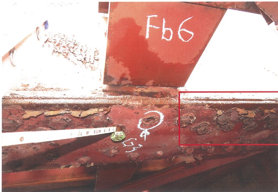
PHOTO 5-14: Missing bolt and loose bolt at the bottom flange of Girder G3 at Floorbeam FB6, looking south. Note the rivets at the bottom flange of Girder G3 exhibit greater than 50% head loss (Rectangle).
