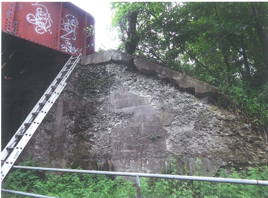
PHOTO 5-18: Large spalls and delaminated concrete throughout the southeast wingwall, looking northeast. Note tree growth behind the wingwall.
