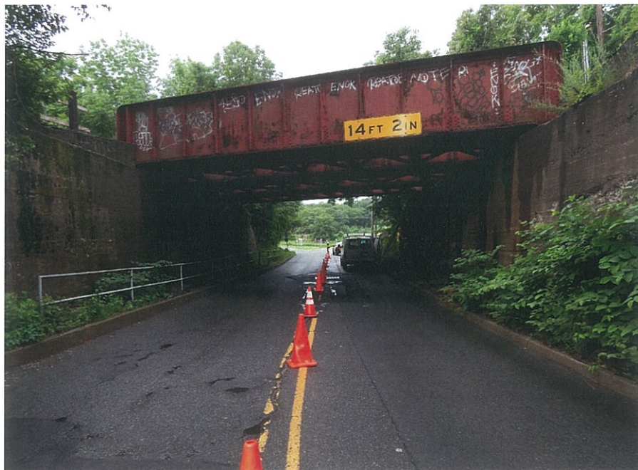
PHOTO 5-2: North elevation, looking south. Work Done: 14'-2" Vertical clearance sign has been installed at the north fascia.
