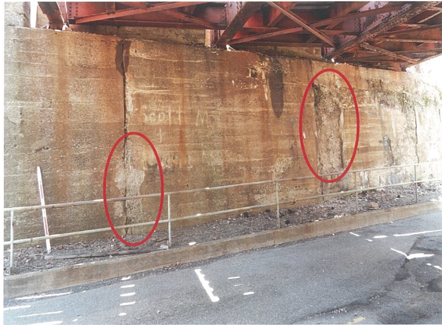
PHOTO 5-7: General view of the east abutment, looking east. Note the large spalls and delaminated concrete throughout the abutment (Circles).
