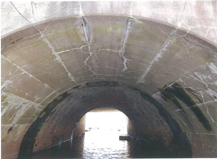
PHOTO 5-7: General view of intrados of concrete and brick arches, looking south. Note several fine cracks with efflorescence, water staining and active water leakage at the concrete arch intrados. Note also, heavy efflorescence throughout the brick arch.
