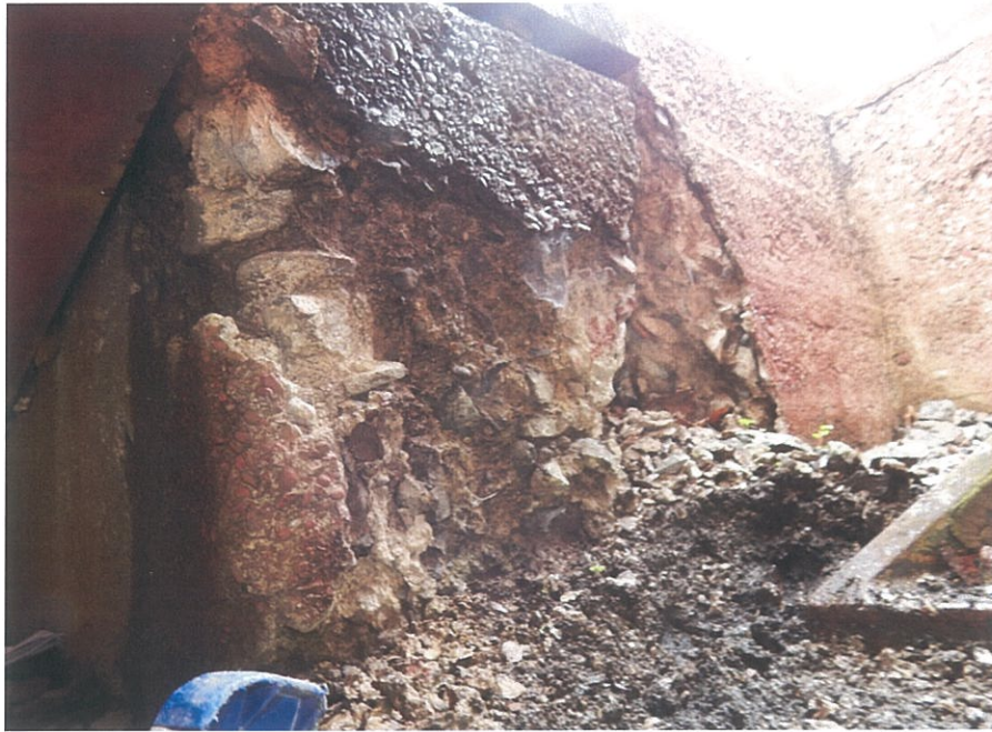
PHOTO 5-19: Large spall and delaminated concrete at the north face of the west abutment backwall adjacent to the Girder G4, looking southwest.
