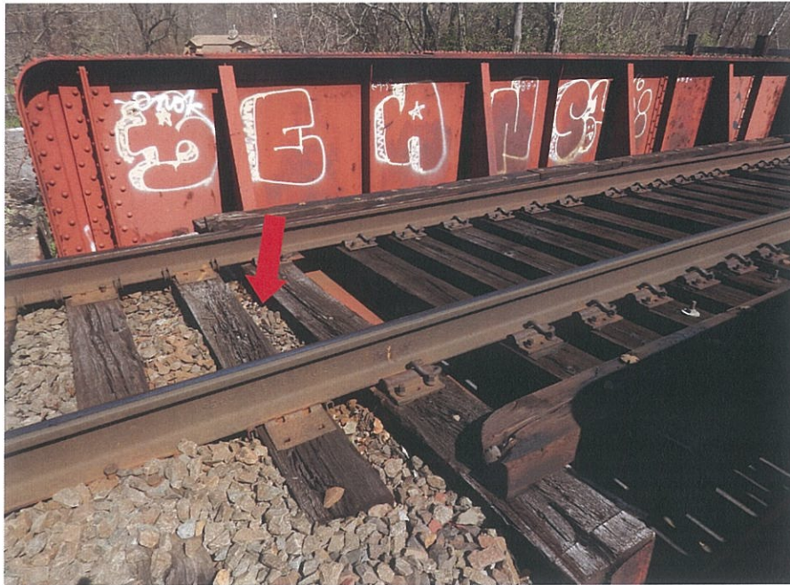
PHOTO 5-9: Decayed ties at the west approach on Track #1, looking northeast. Note low ballast adjacent to the bridge (Arrow) and graffiti at the web plate of Girder G4.
