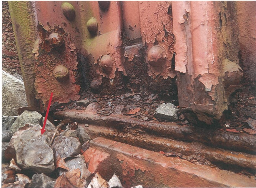
PHOTO 5-17: Missing sole plate bolt at the north side of Girder G3 bearing over the east abutment, looking southeast. Note the accumulation of ballast on the bearing seat.
