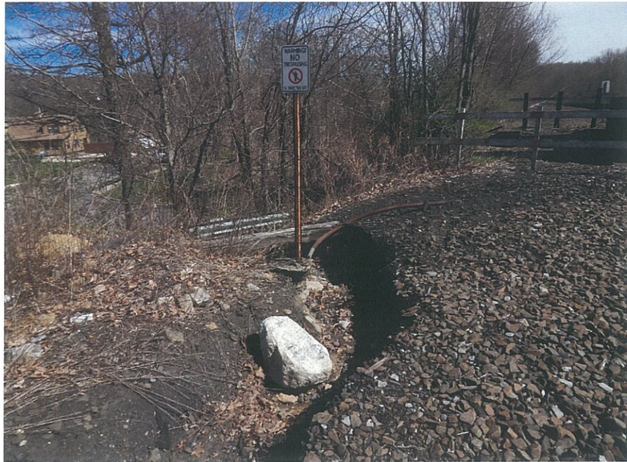
PHOTO 5-21: Erosion hole at the northwest approach embankment, looking northeast.
