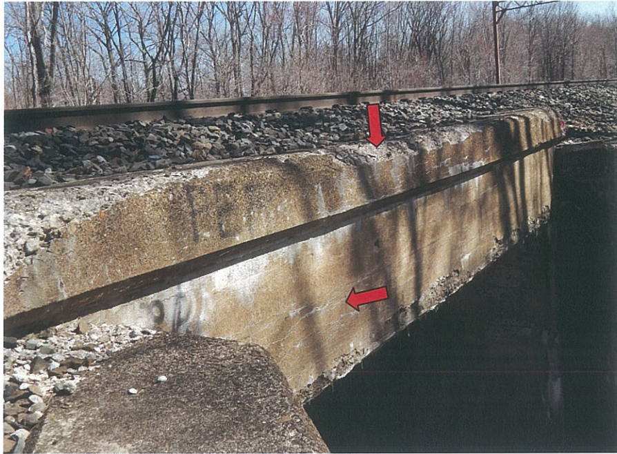
PHOTO 5-9: Spalled and or delaminated concrete throughout the top of south headwall, looking northeast. Note fine cracks with efflorescence at random locations of the headwall.
