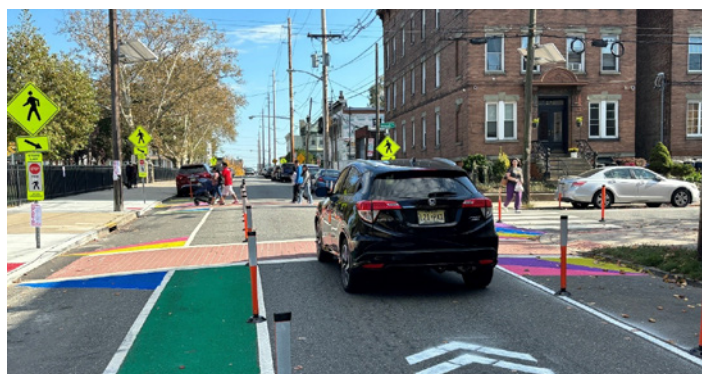
Figure 22: An example demonstration project in Jersey City that included painted bike lanes, curb extensions, flexible delineators, and a chicane. (Image Source: Stantec)
