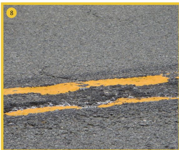
The centerline rumble strip is worn
