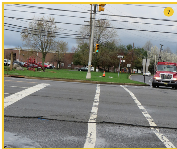
Pavement markings are faded
