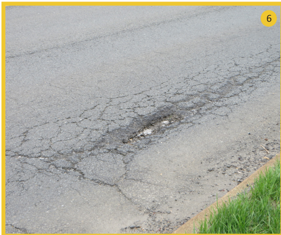
Pavement condition is lacking
