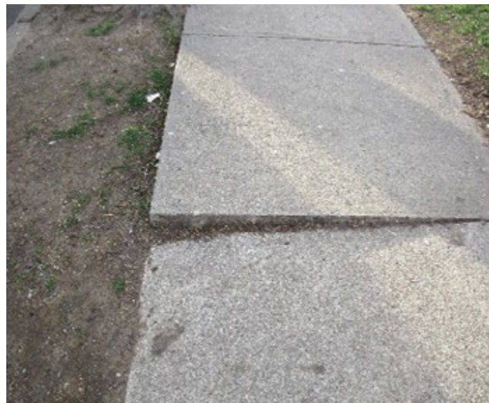
FIGURE 15. UNEVEN PAVEMENT ALONG THE PARK'S WESTERN PERIMETER.
