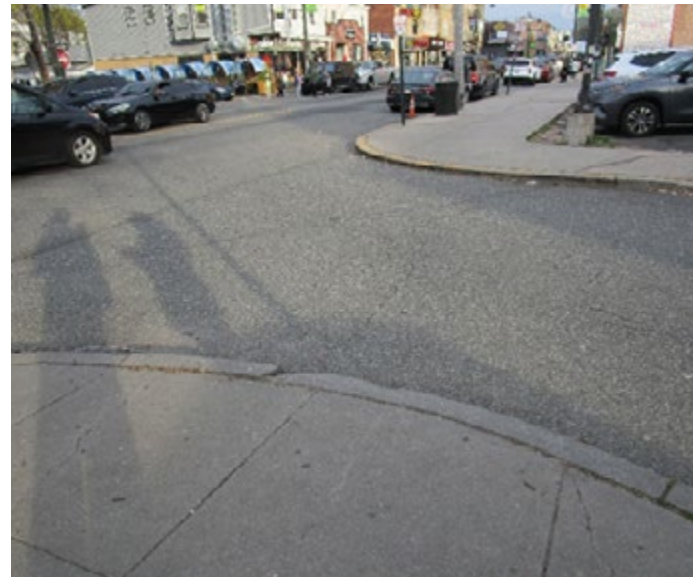
FIGURE 16. PEDESTRIANS CROSS PACIFIC STREET WITHOUT A PAINTED CROSSWALK OR ADA CURB CUT.
