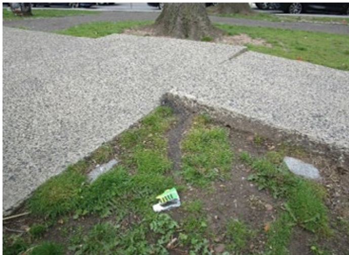
FIGURE 7. SOME SEGMENTS OF THE PARK'S WESTERN SIDEWALK ARE UNEVEN AND PRESENT A TRIP HAZARD.
