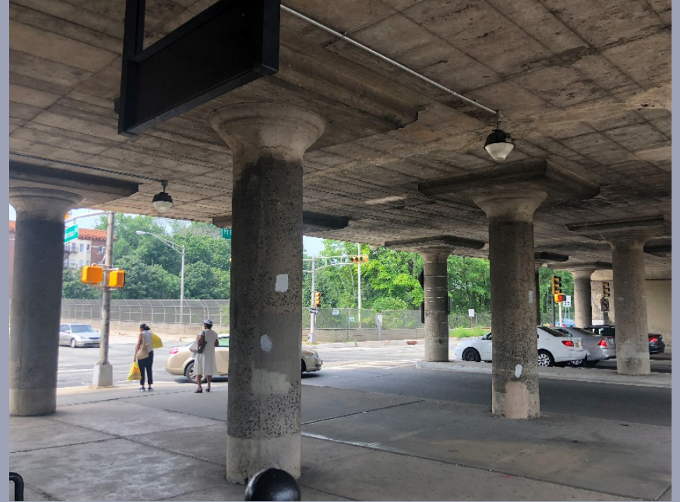
View from the staircase to South Harrison Street. The underpass and arcade are generally sufficiently lit by natural light during the day.
