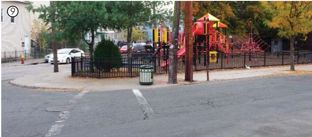
Crosswalks, like this one at the neighborhood playground, are in need of fresh paint & better crossing signalization
