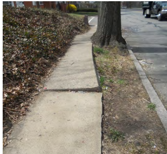
Cracked sidewalks are frequent along Irvington Avenue
