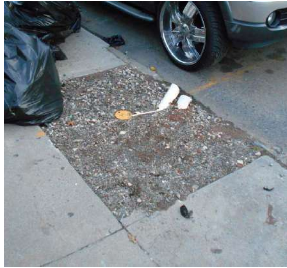
Image 38 Broken Sidewalk on East Jersey Street
