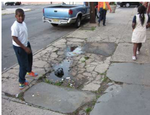
Image 12 Damaged Sidewalk on 3rd St
