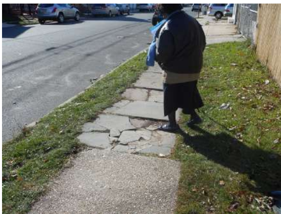
Image 60 Broken sidewalk on Geneva Street
