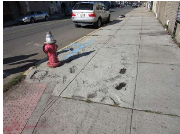
Image 45 Vandalized sidewalk on 1st Street
