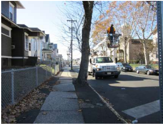
Image 52 Uprooted Sidewalk on Delaware Avenue
