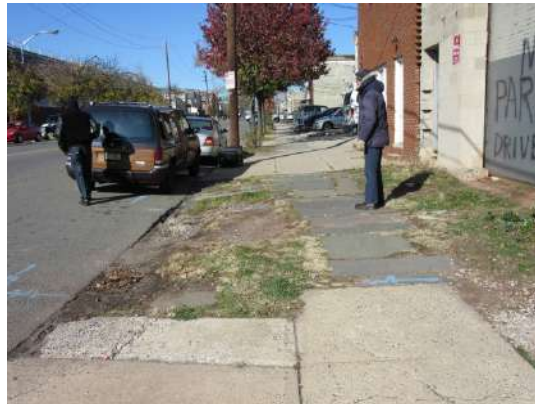
Image 49 Broken sidewalks between 1st and 2nd
