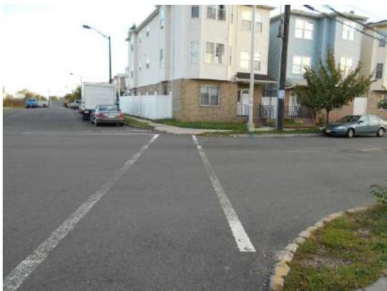
Image 39 Faded crosswalk striping
