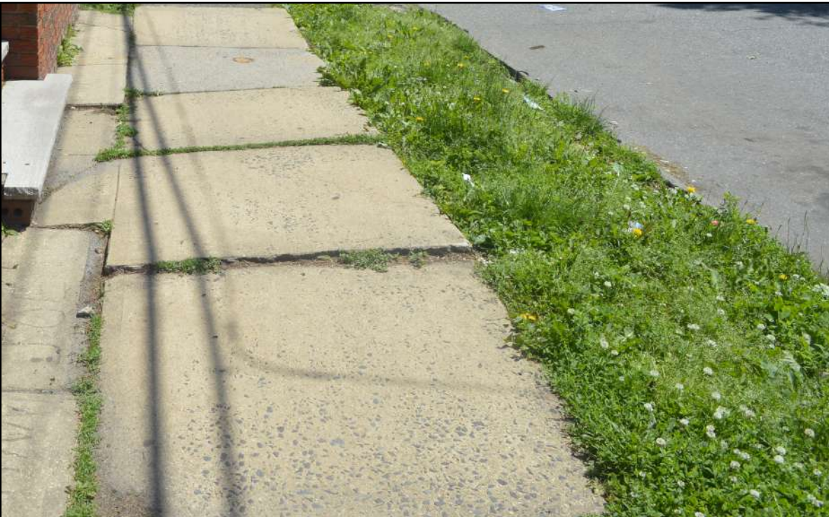
Uneven sidewalk on Elm Street.
