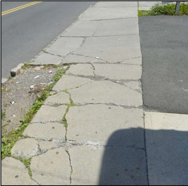
Cracked sidewalk on Orchard Street.
