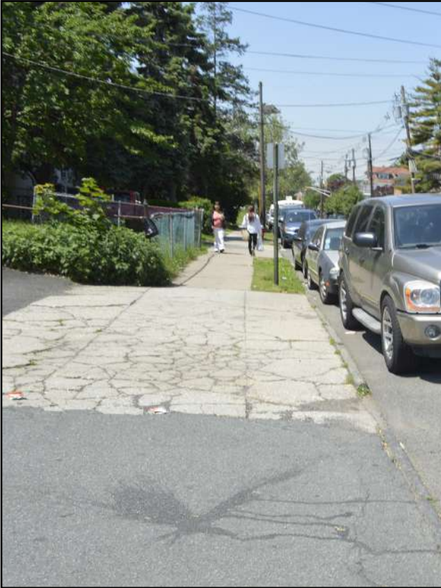
Cracked sidewalk on Stiles Street.
