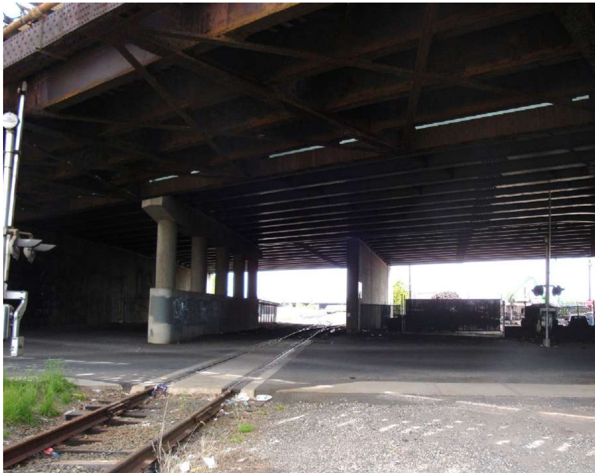
Lack of lighting and pedestrian amenities under East Ferry's overpasses limit walking and biking opportunities.
