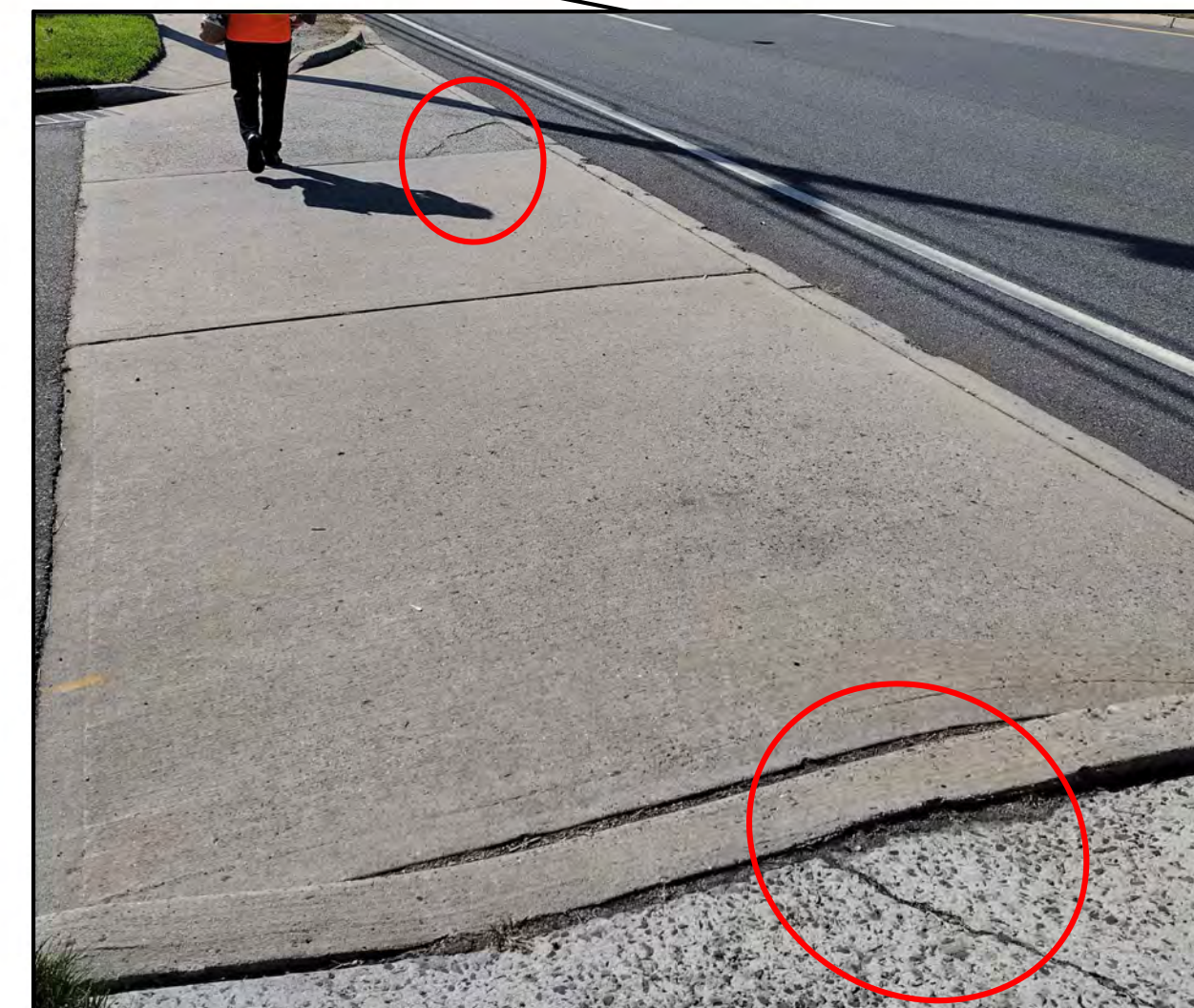
Cracked sidewalk and driveway
