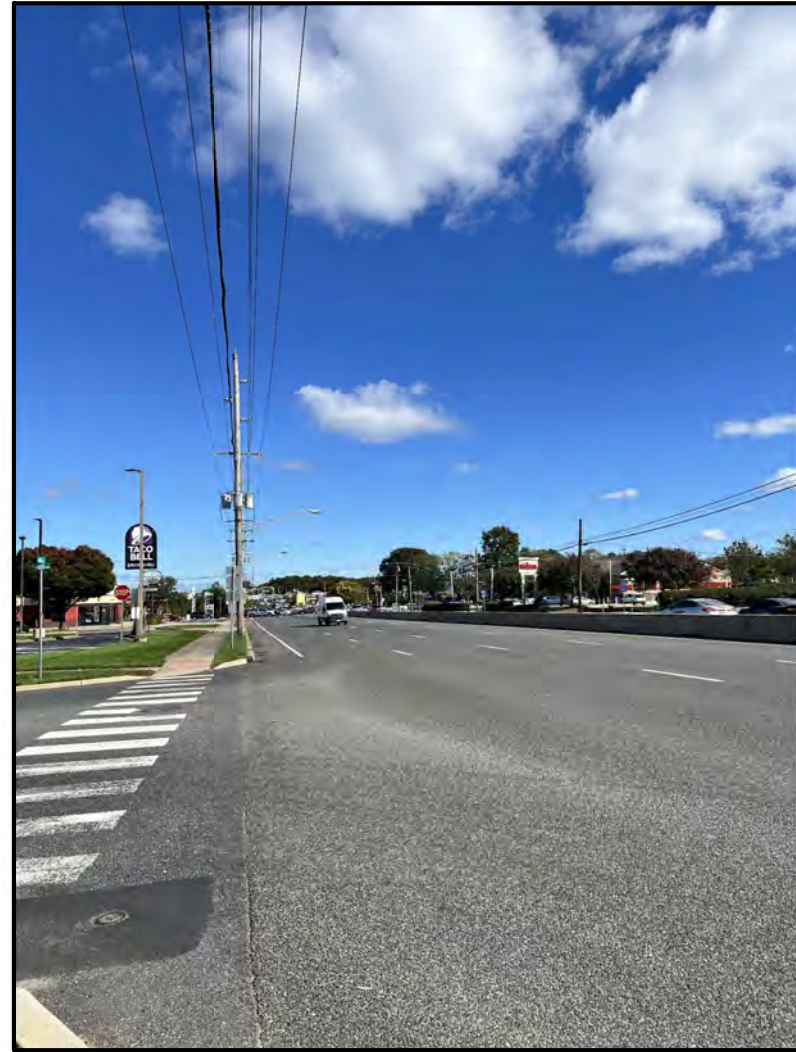
No pavement markings to indicate lane ends and merges
