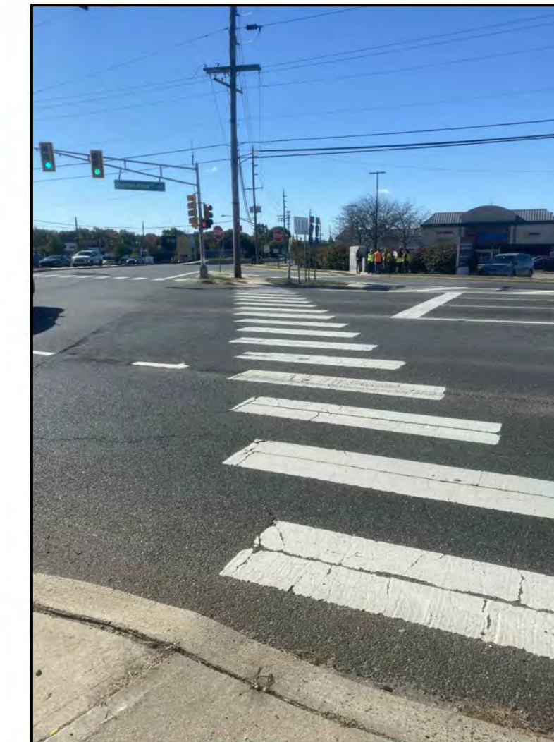
Crosswalk Striping needs to be revised
