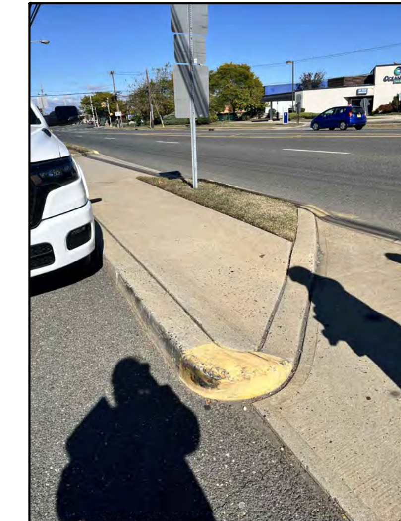
Curb ramps not ADA compliant
