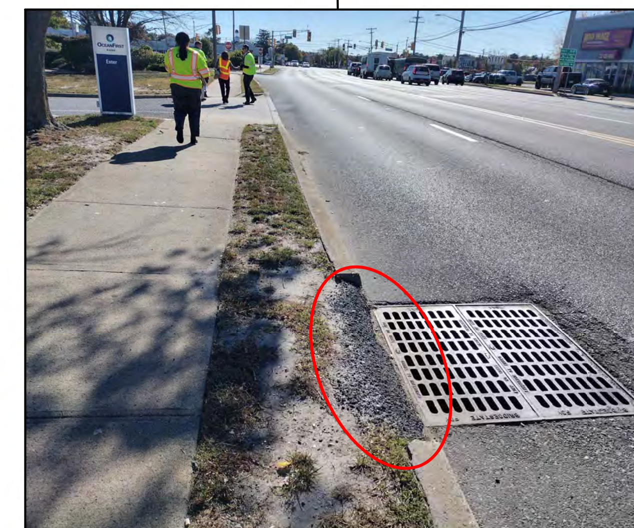
Broken off Curb
