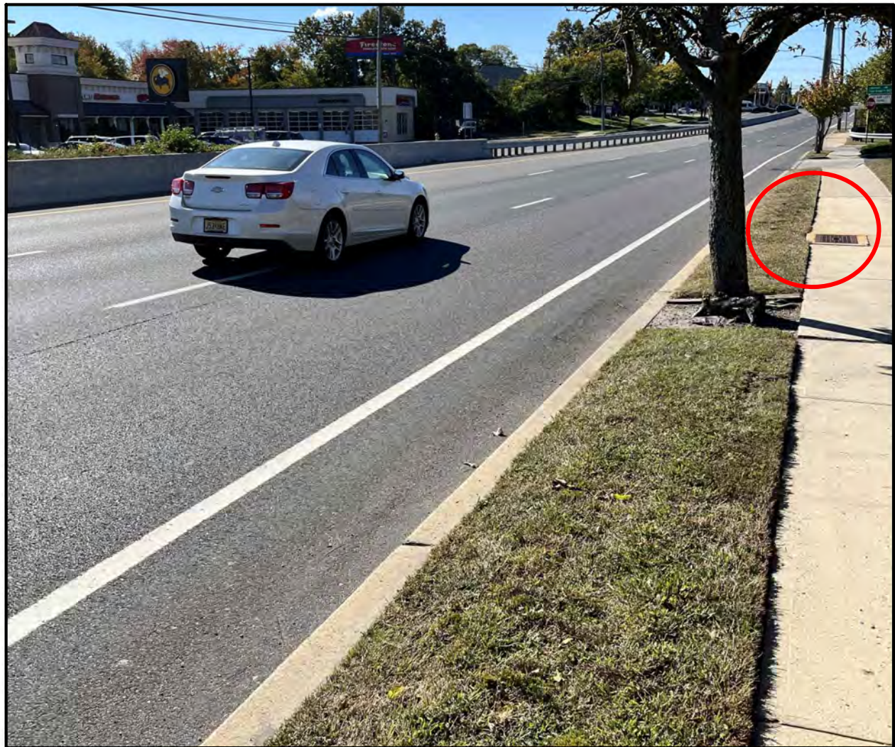
Junctionbox not flush with sidewalk and is a tripping hazard
