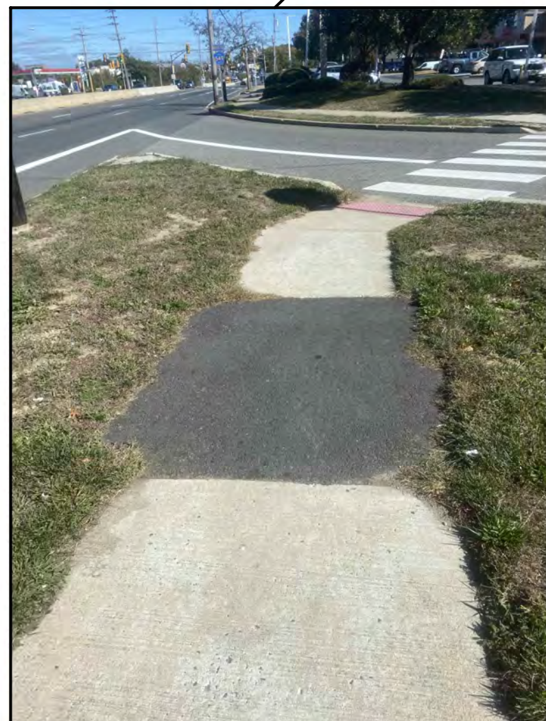
Sidewalk is not consistently concrete
