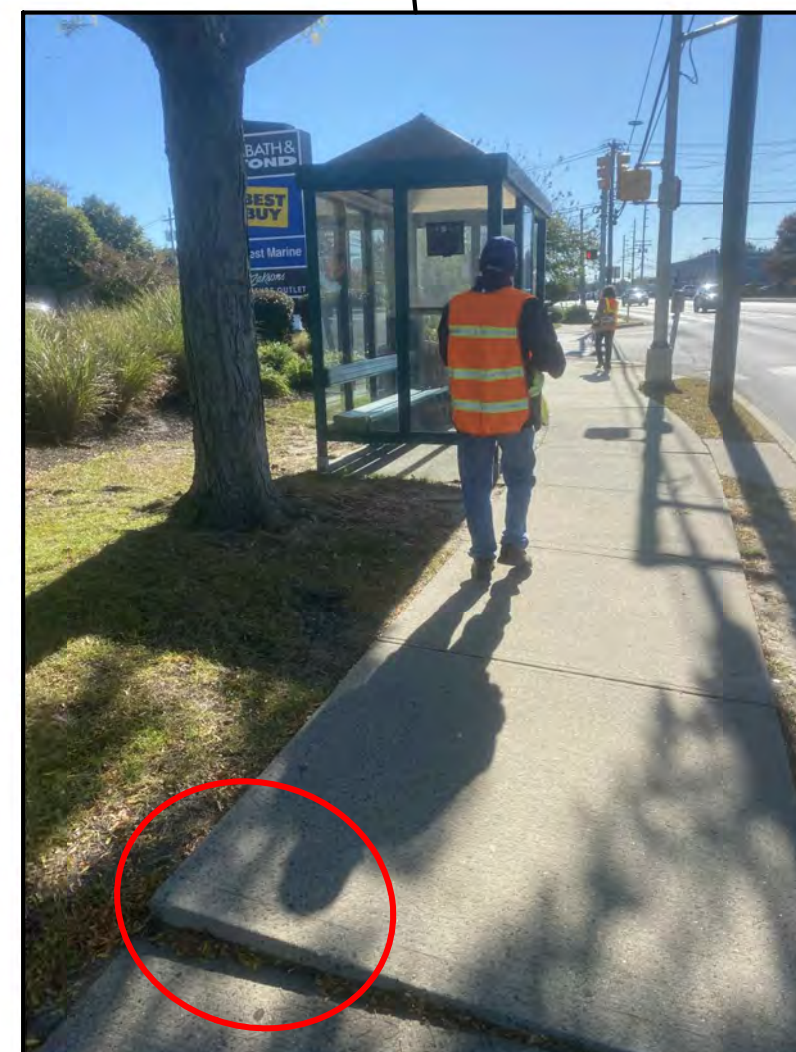
Tripping hazard due to uneven sidewalk
