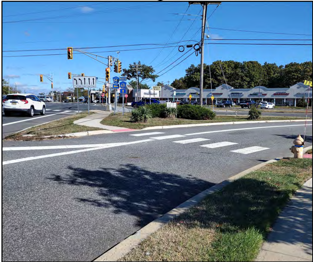
Cracked Crosswalk and shoulder paint
