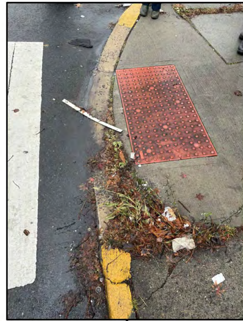
Vegetation and Ponding at the curb ramp
