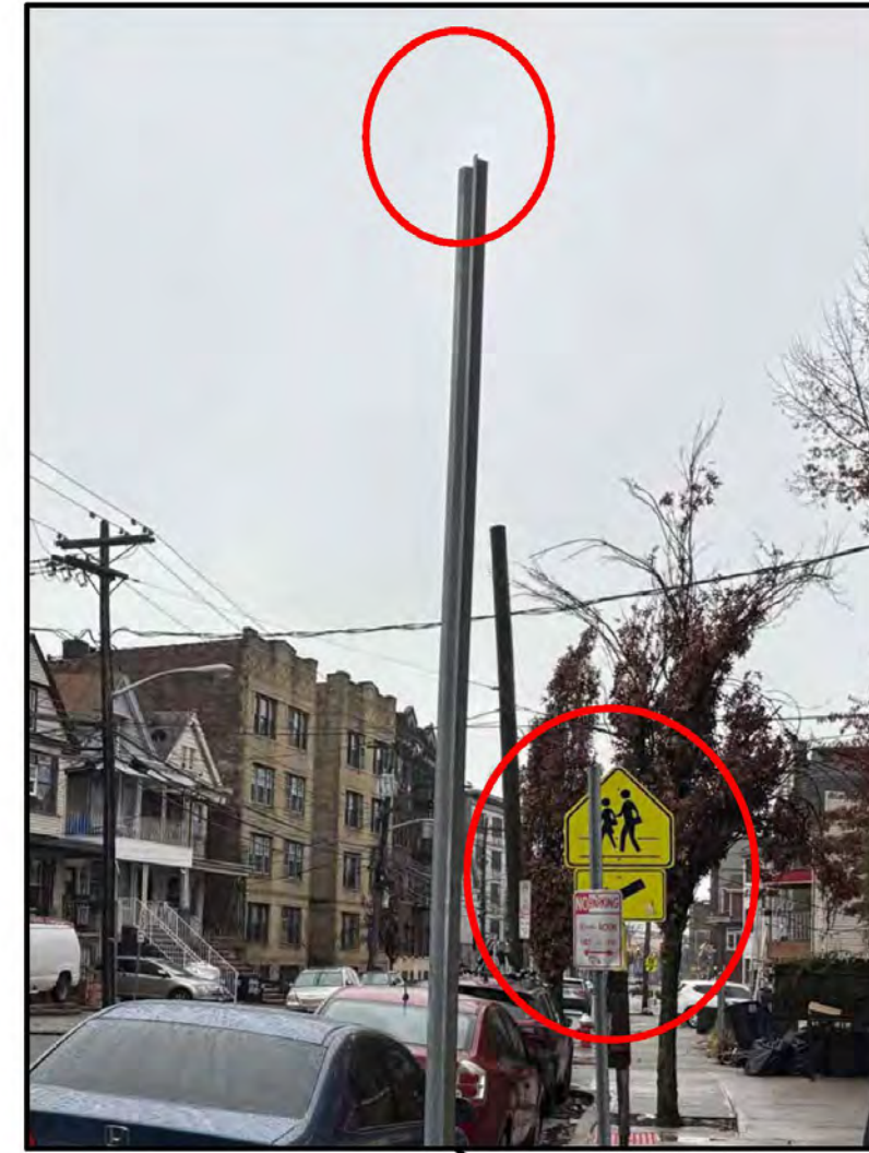
Missing sign; signs mounted lower than required
