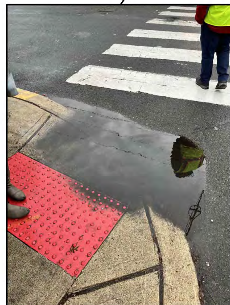
Ponding at the curb ramp
