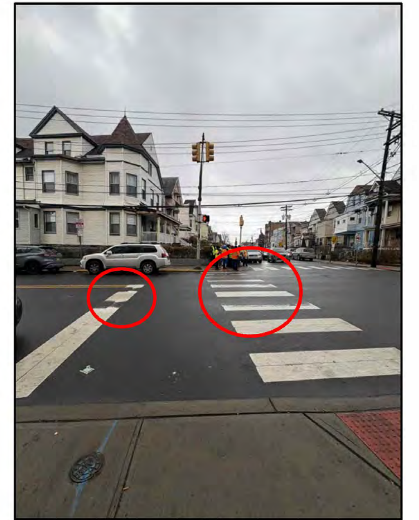
Faded stop bar striping; faded crosswalk striping
