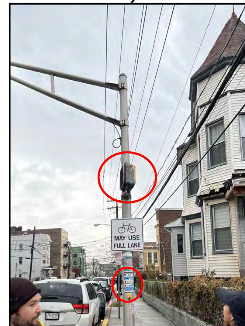
Worn signal equipment; damaged push button sign
