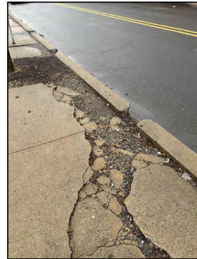
Cracked and damaged sidewalk and curb
