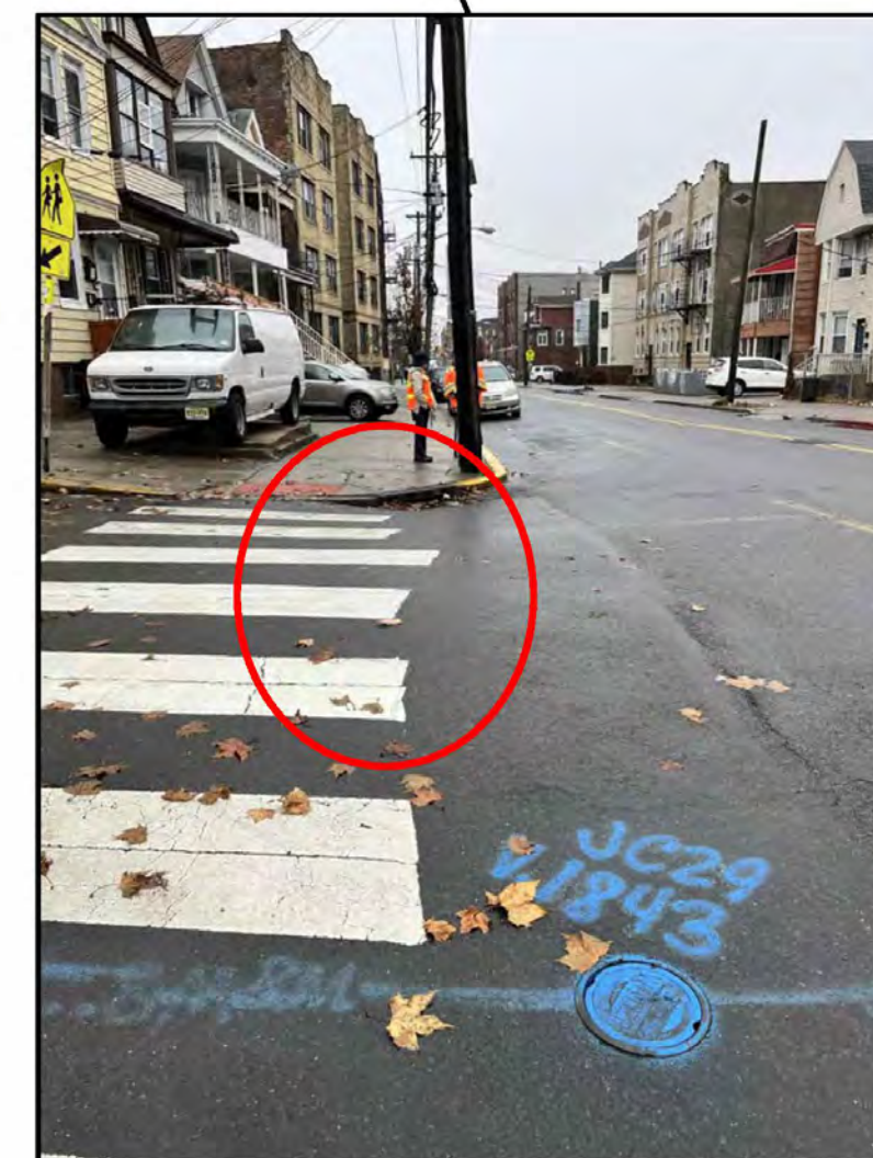
Crosswalk striping is not straight; Curb ramp is not flush with the road
