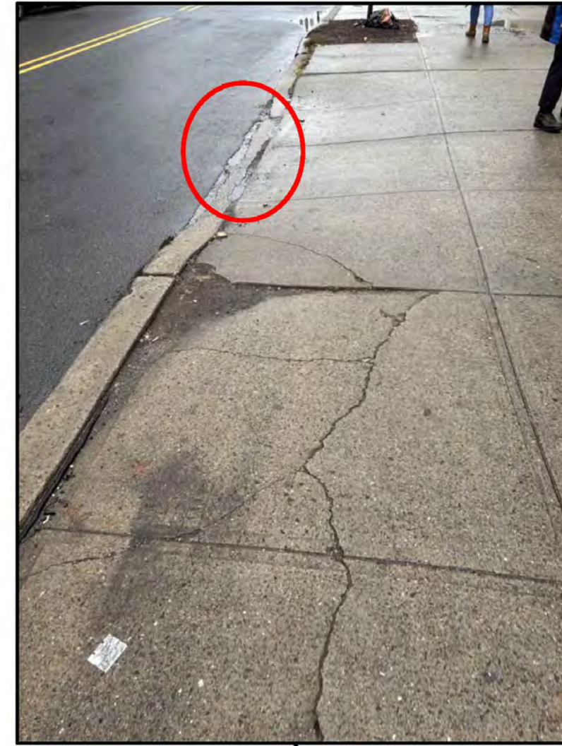
Cracked sidewalk; Broken driveway curb
