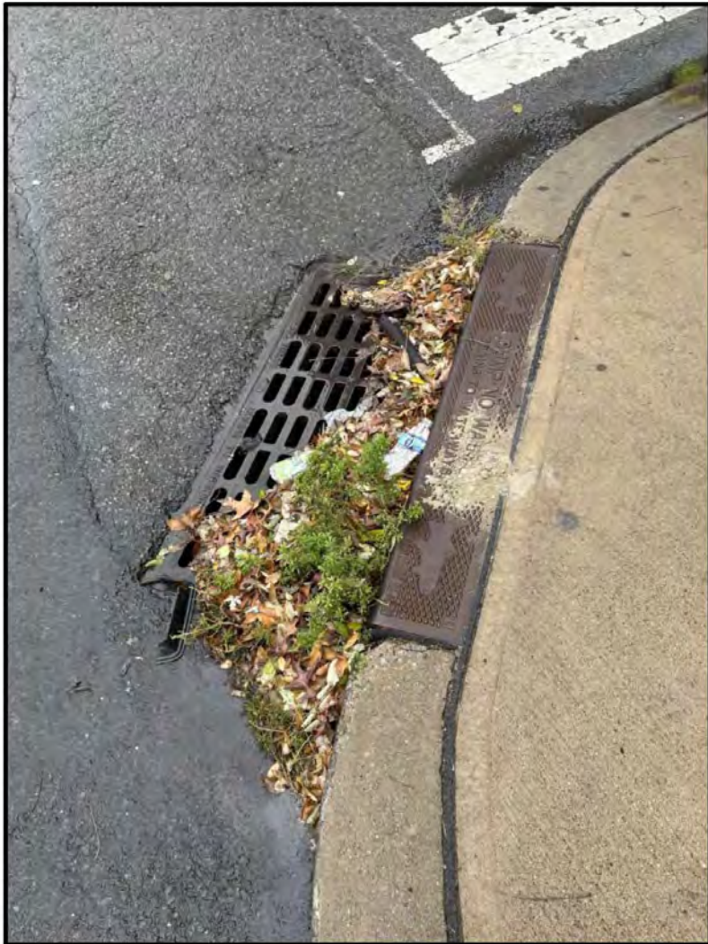
Vegetation blocking the inlet
