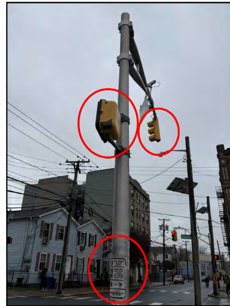
Outdated signal equipment; damaged push button sign
