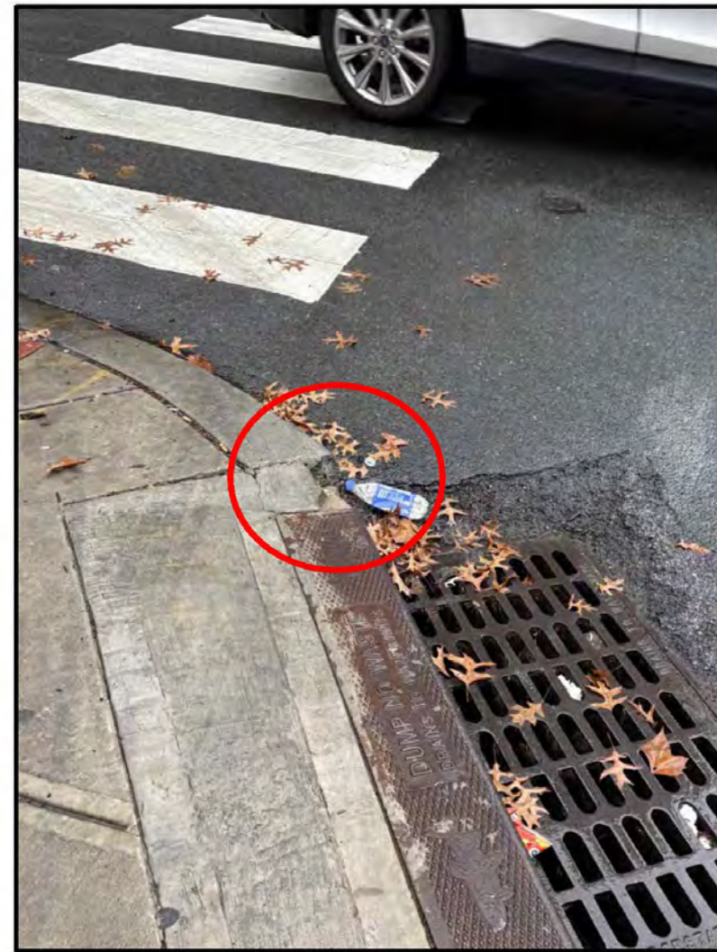
Broken curb around the inlet
