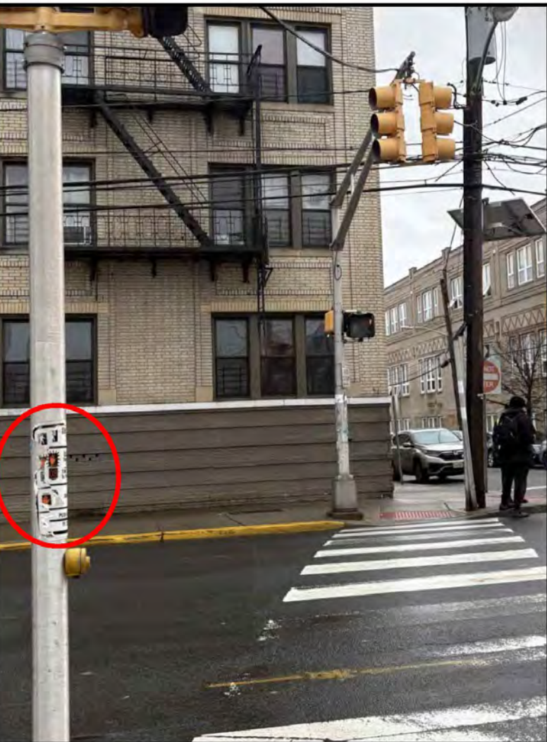
Faded crosswalk; faded pedestrian crossing sign
