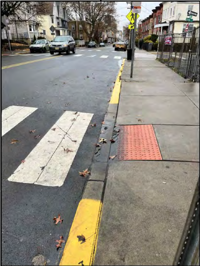
Ponding at the curb ramp
