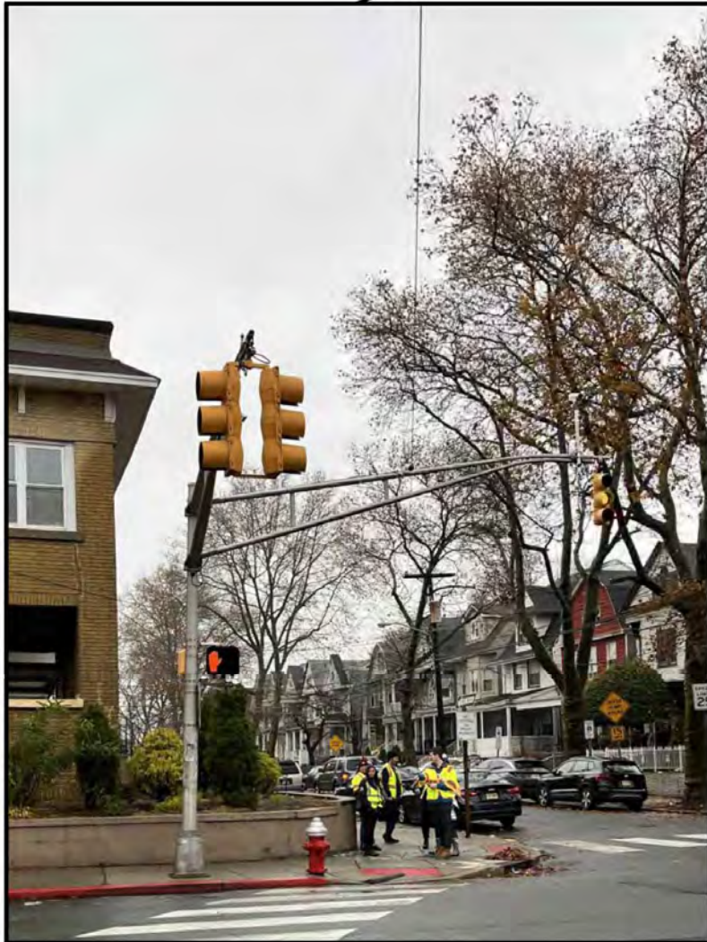
Outdated signal equipment
