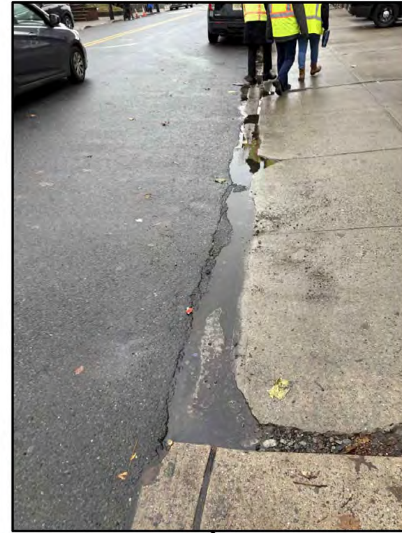
Broken driveway concrete; ponding at the end of the driveway
