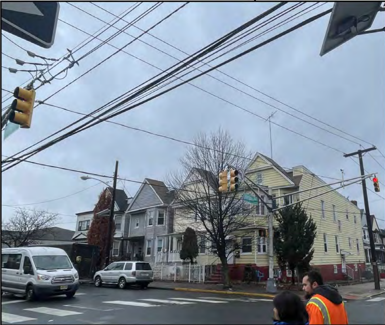
Outdated signal equipment
