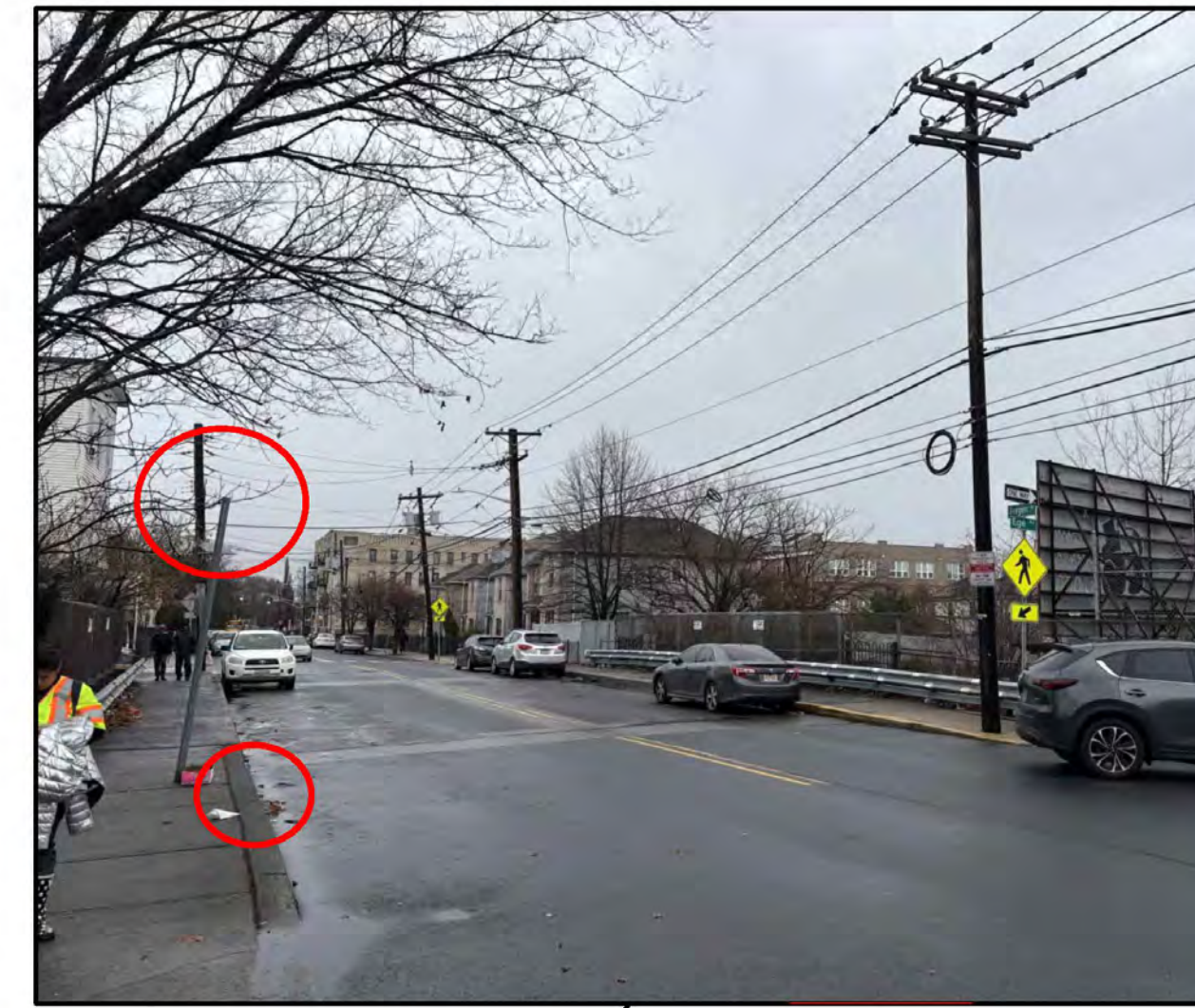
Missing crosswalk striping, crosswalk sign and ADA curb ramp
