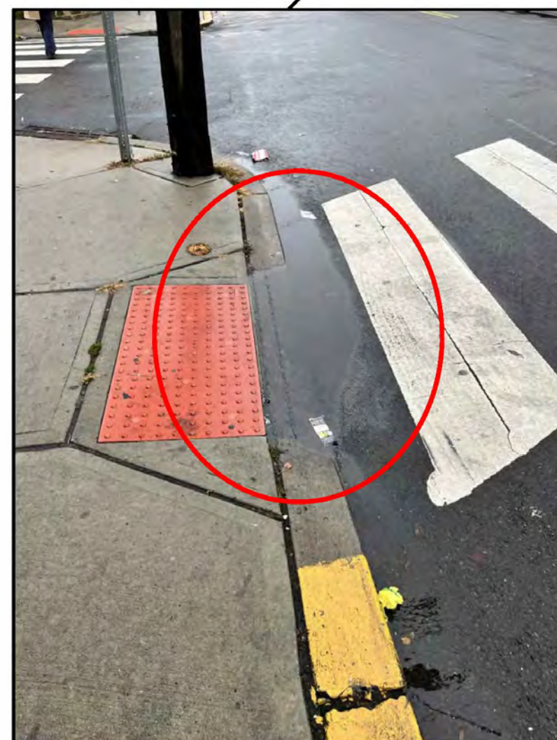
Ponding at the curb ramp
