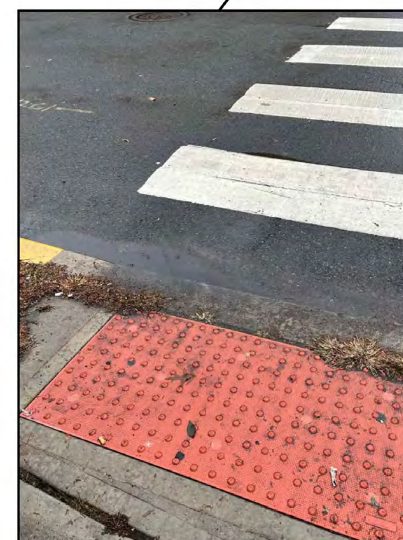
Ponding at the curb ramp
