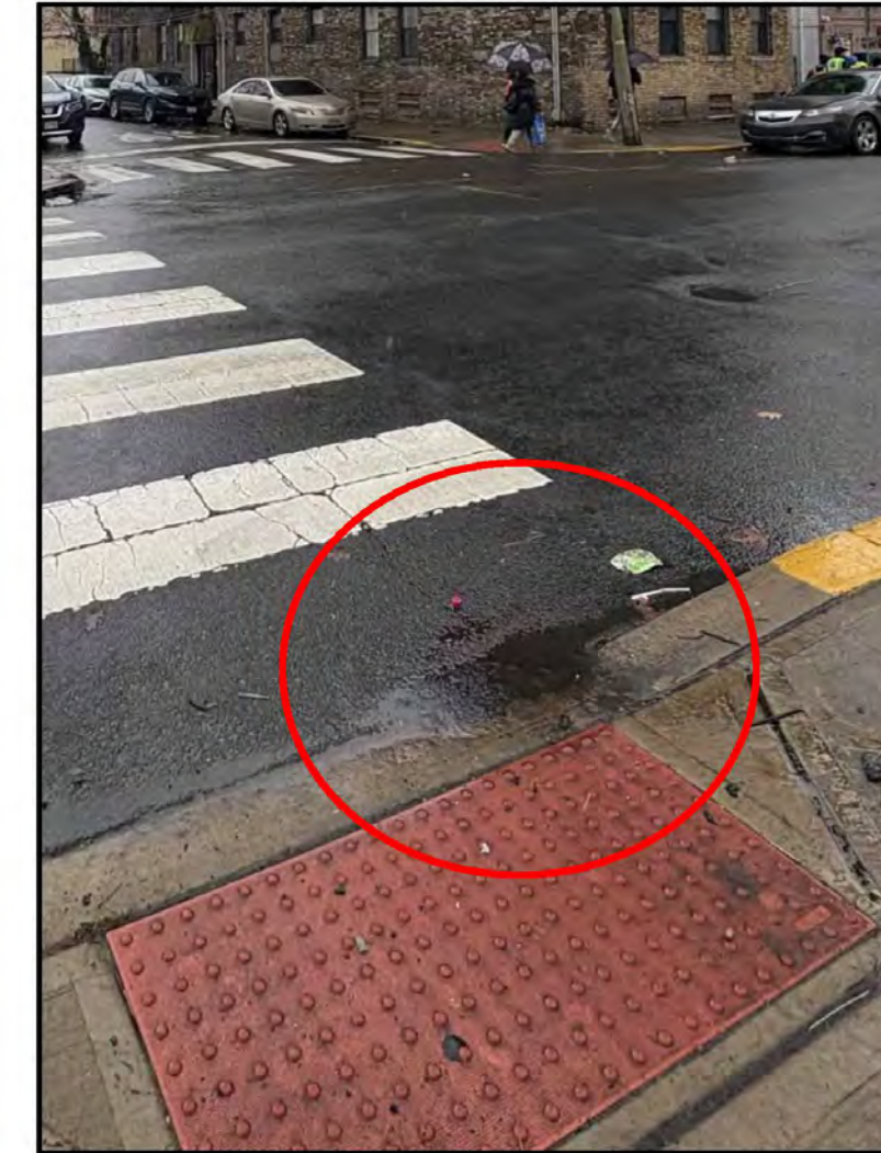
Ponding at the curb ramp
