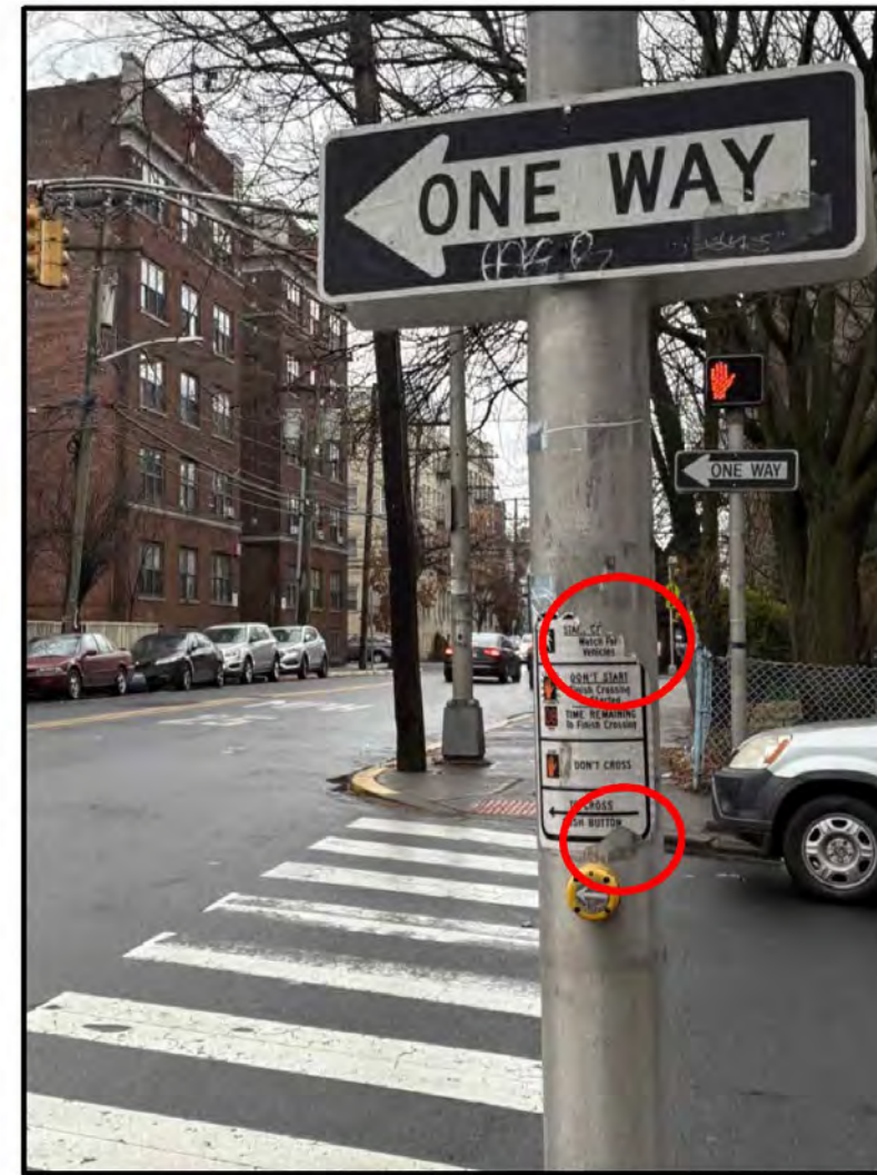
Cracked and vandalized sign; damaged push button sign
