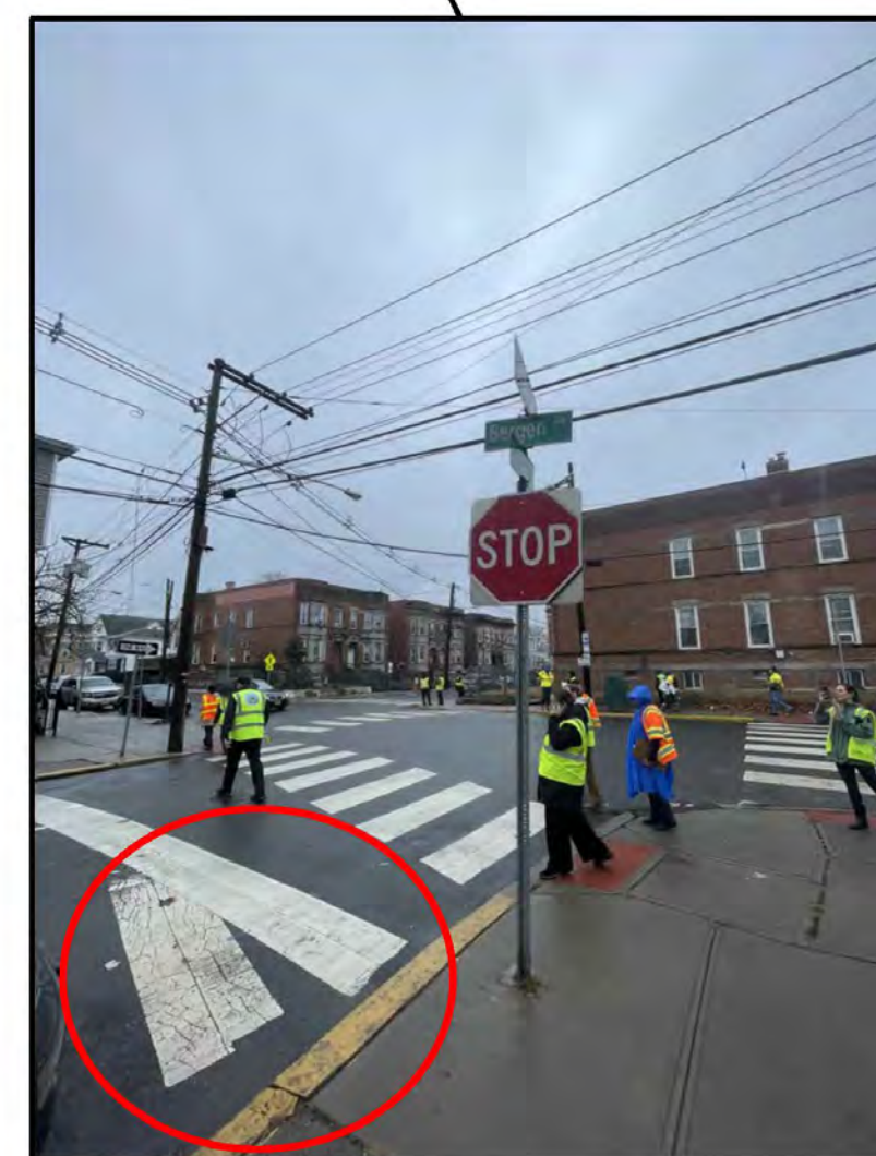
Conflicting stop bar striping
