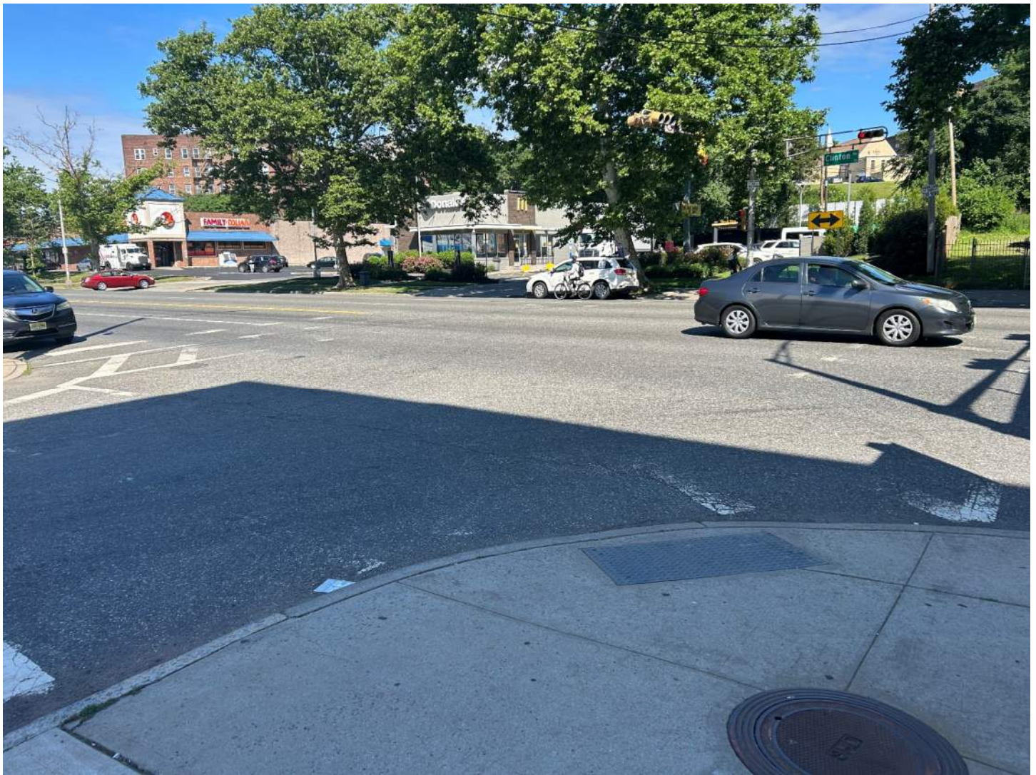
Photo #5: Worn Crosswalk Striping
