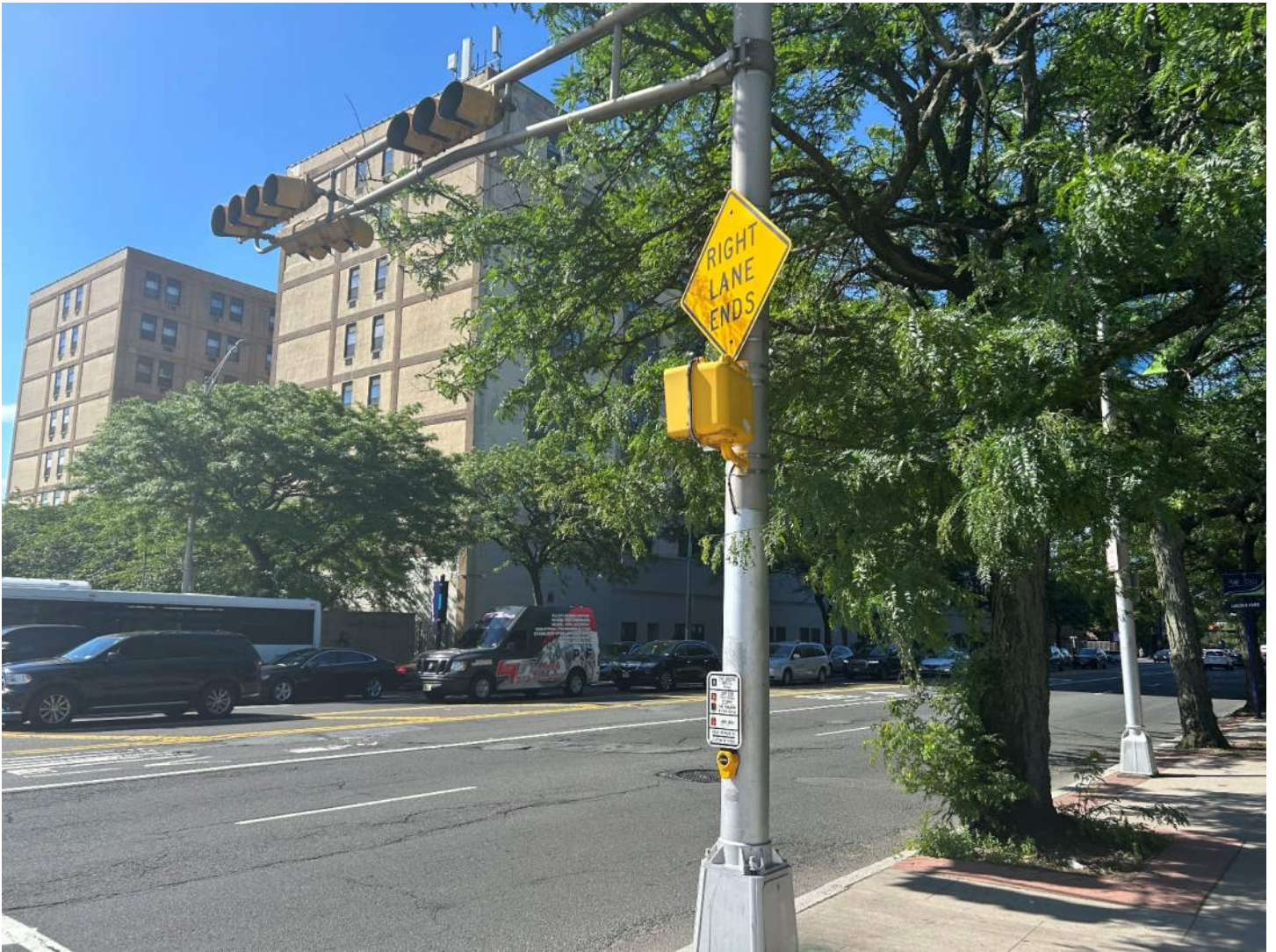
Photo #6: Outdated Signal Equipment
