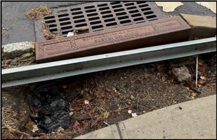
Pot hole adjacent to the sidewalk
