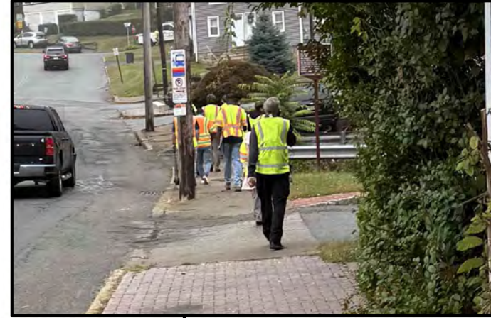
Non-ADA compliant bus stop; Broken curb; No buffer between vehicular lane and sidewalk
