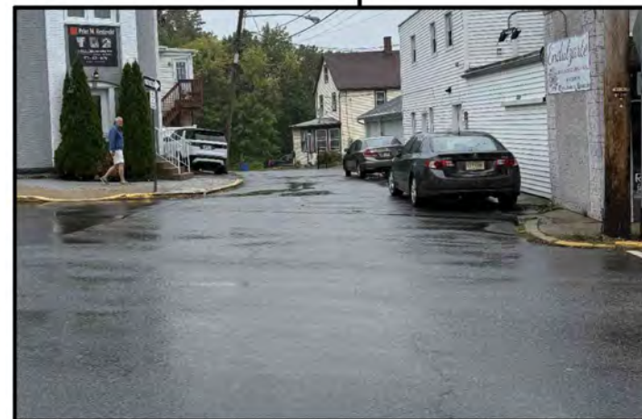
No crosswalk; Missing ADA curb ramps
