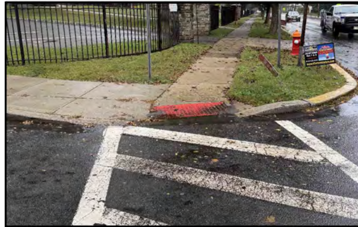
Water accumulation at the curb ramp; Faded crosswalk
