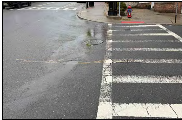
Faded crosswalk; Inconsistent sidewalk width due to the fire hydrant
