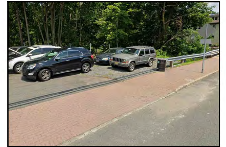
No ADA compliant curb ramp to detect the driveway apron; No driveway warning sign
