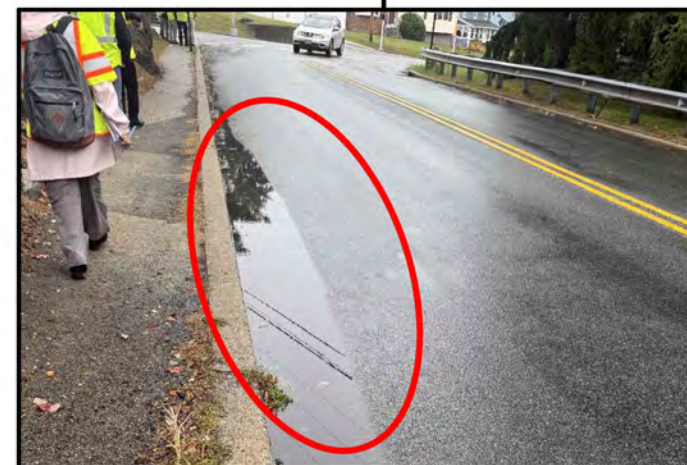
Water accumulation issues; No sidewalk on the SB edge
