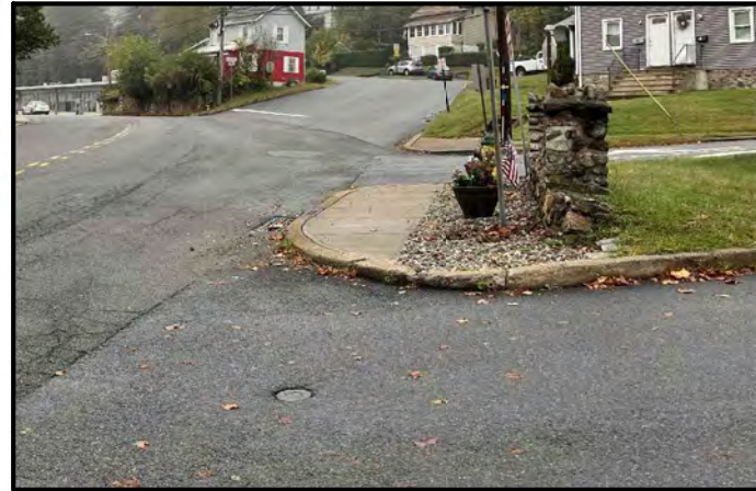
No ADA compliant curb ramp; No sidewalk and crosswalk
