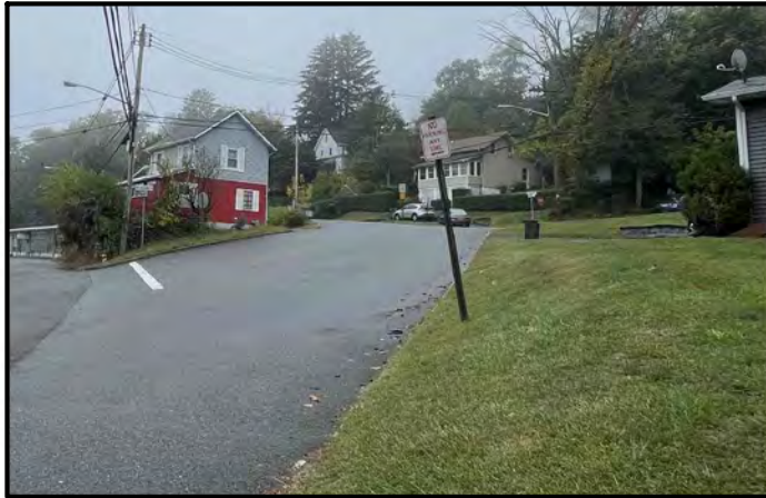
No edgeline; No centerline; Missing ADA compliant ramps, sidewalk and crosswalk
