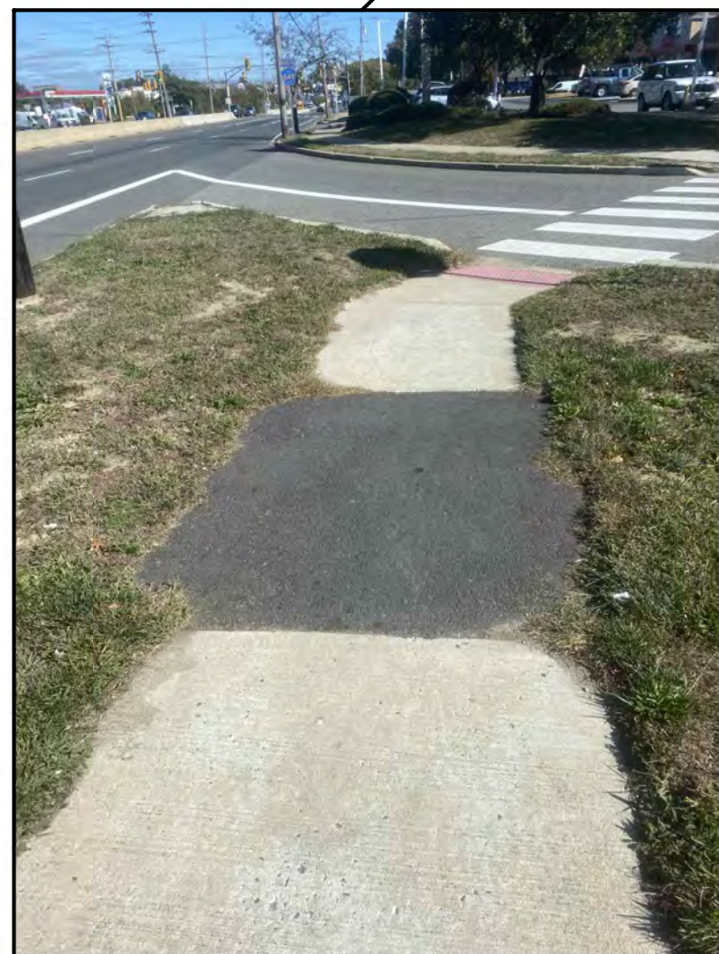
Sidewalk is not consistently concrete
