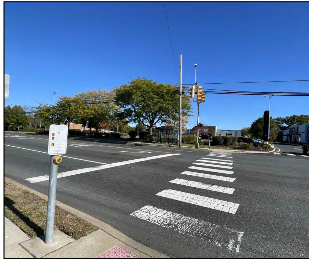
Worn Crosswalk paint
