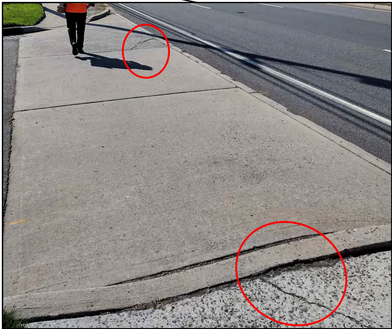
Cracked sidewalk and driveway
