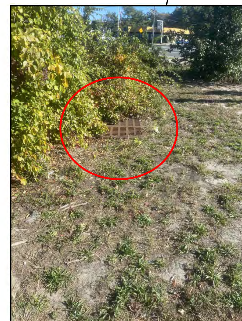
Drain is not at the lowest point and is blocked by overgrown vegetation
