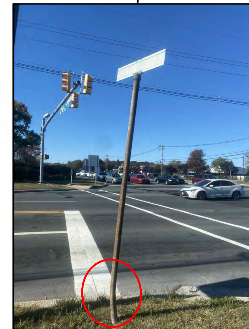
Signage pole is damaged
