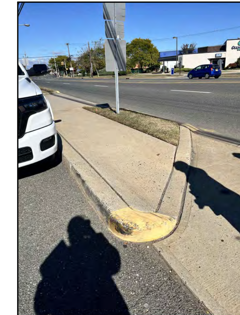
Curb ramps not ADA compliant
