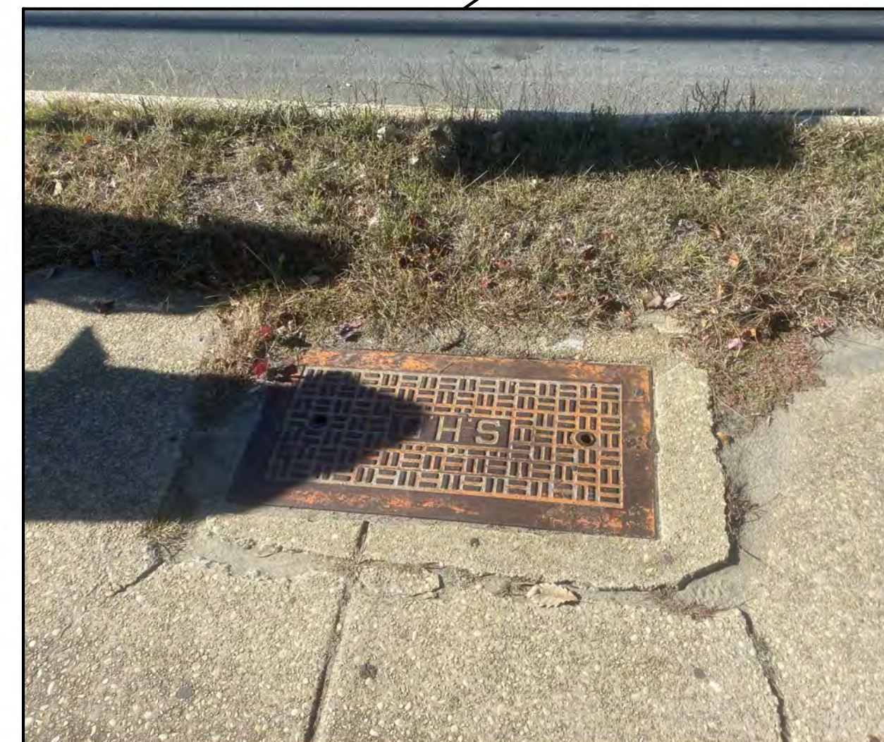
Broken sidewalk around the junction box
