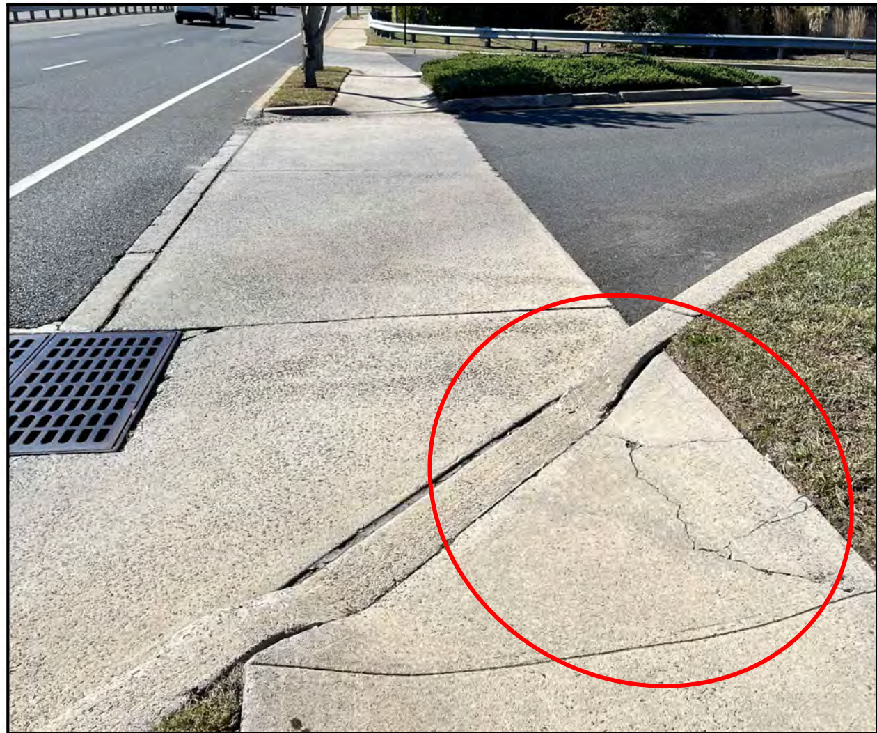
Cracked curb ramp; Ramp is not ADA compliant
