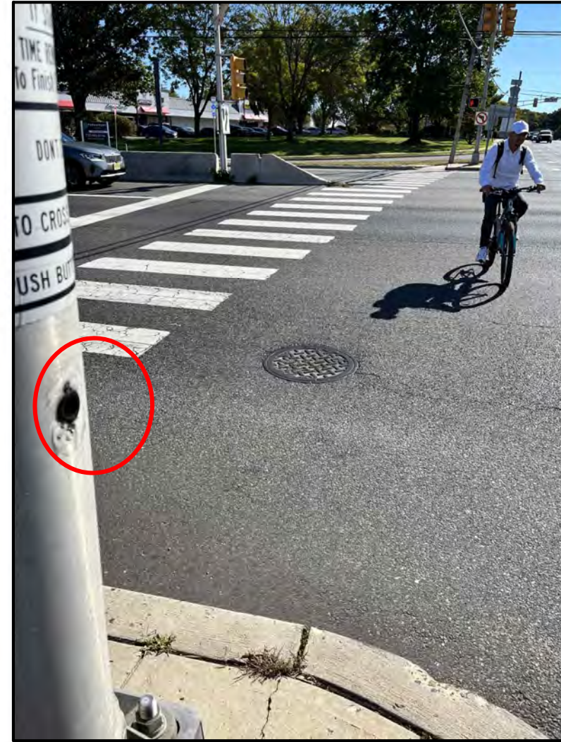
Missing pedestrian push button; Bicyclist crossing adjacent to the crosswalk
