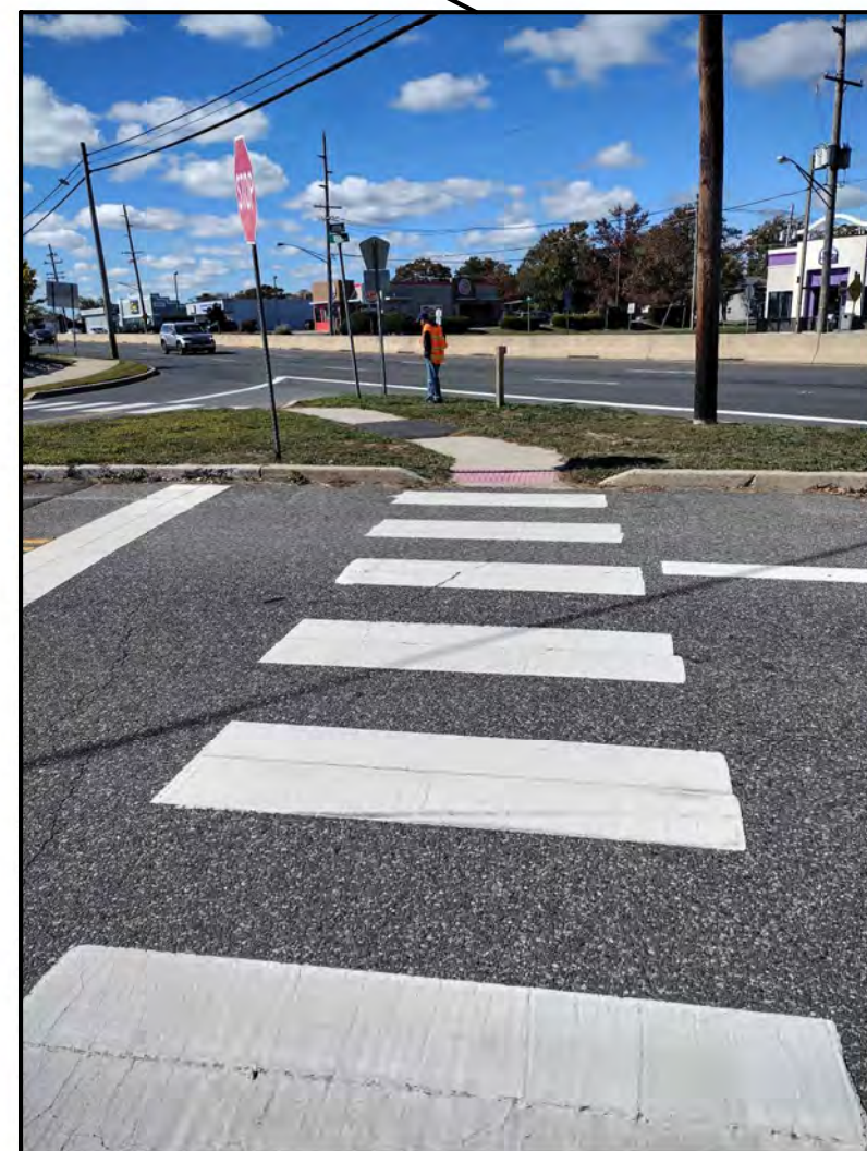
Stop bar is set too far back to have visibility of Brick Boulevard NB traffic
