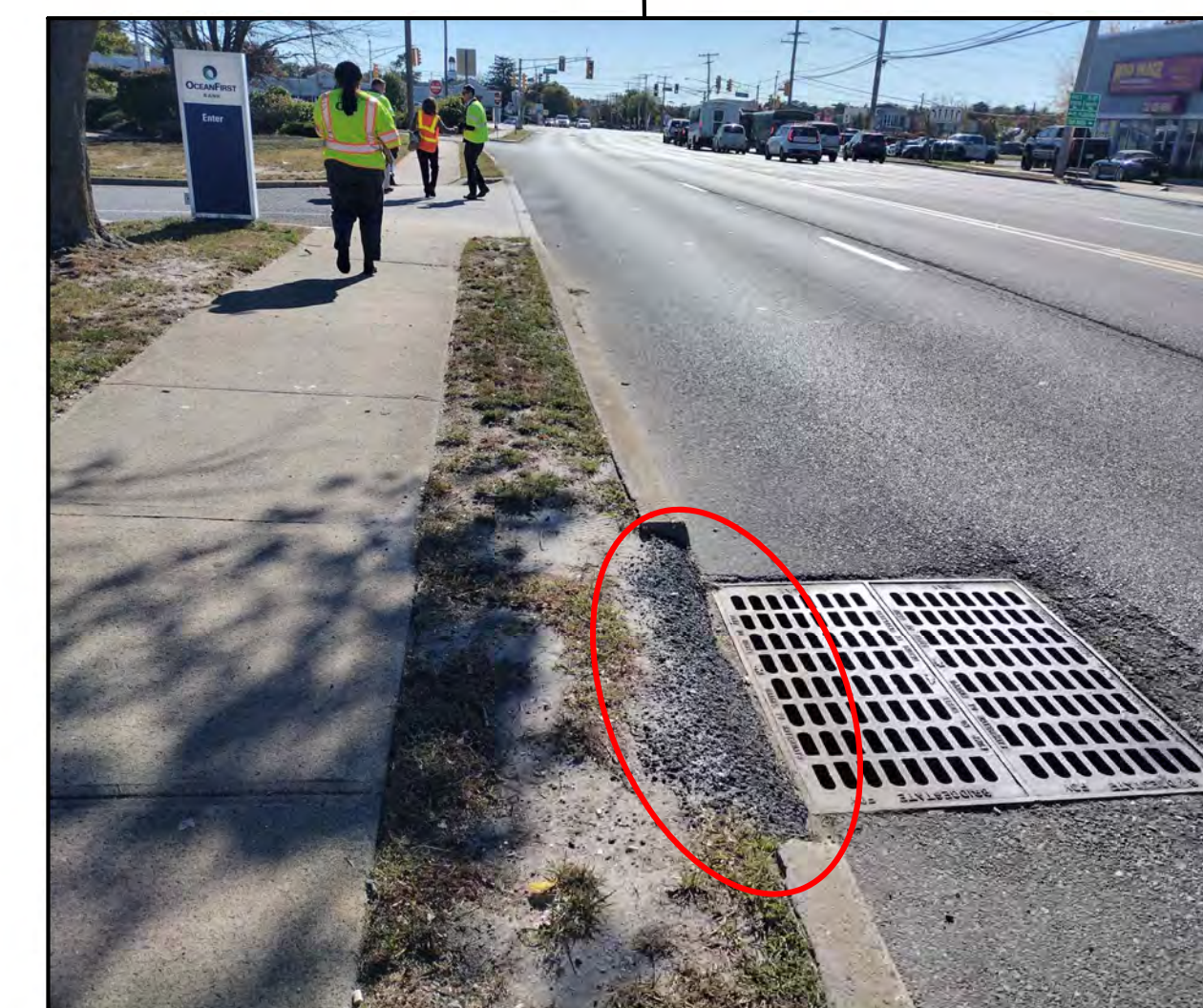
Broken off Curb
