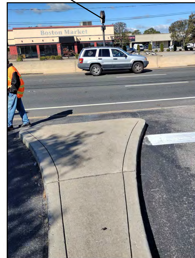
Raised island is not ADA compliant
