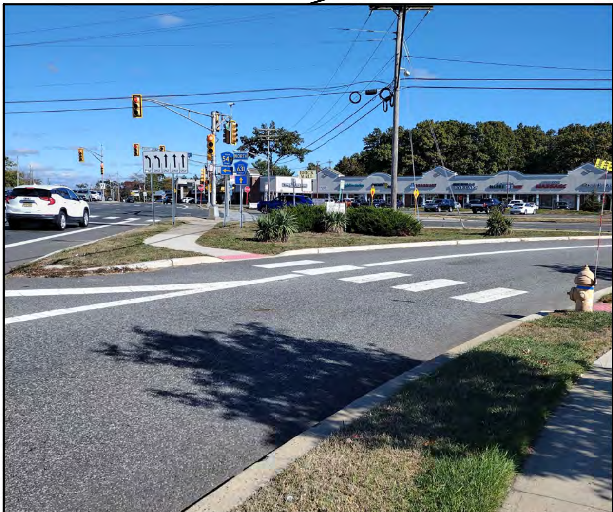
Cracked Crosswalk and shoulder paint
