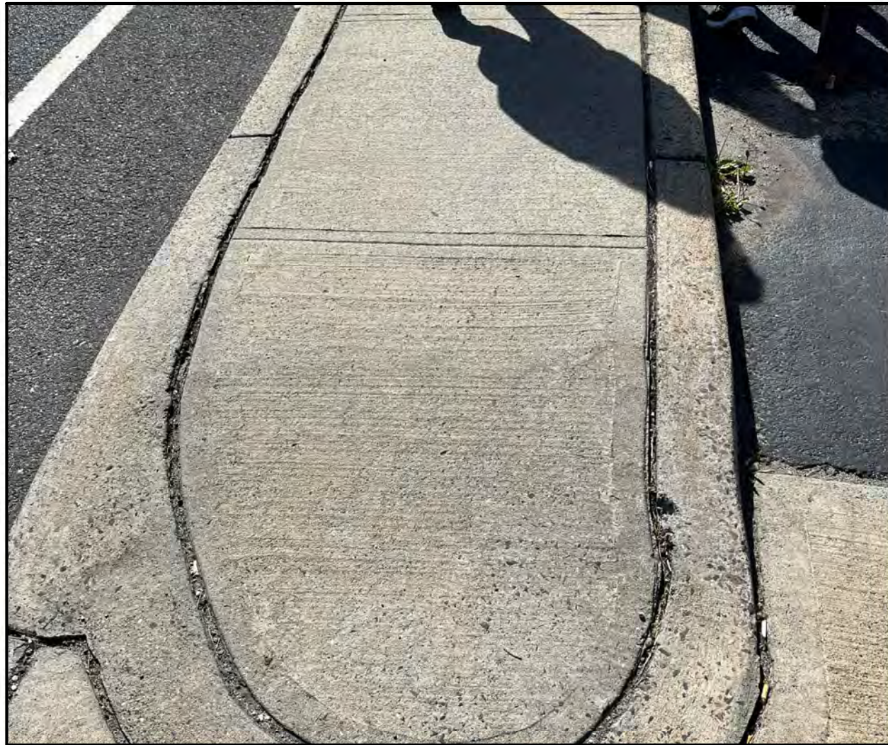
Sidewalk not ADA compliant and not up to size standards
